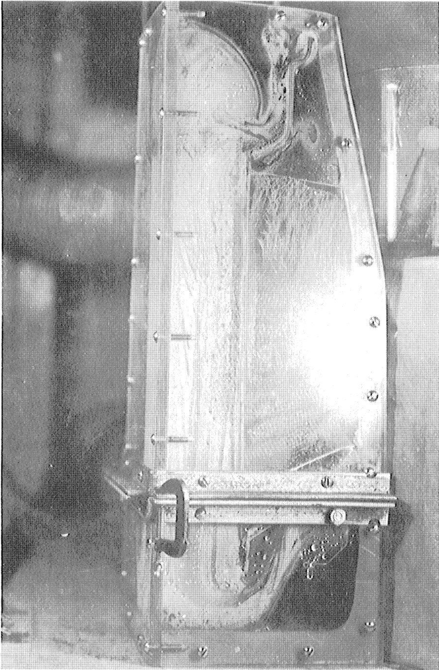
Figure 10. Flow path through air cleaner shown by steam condensate on window.
