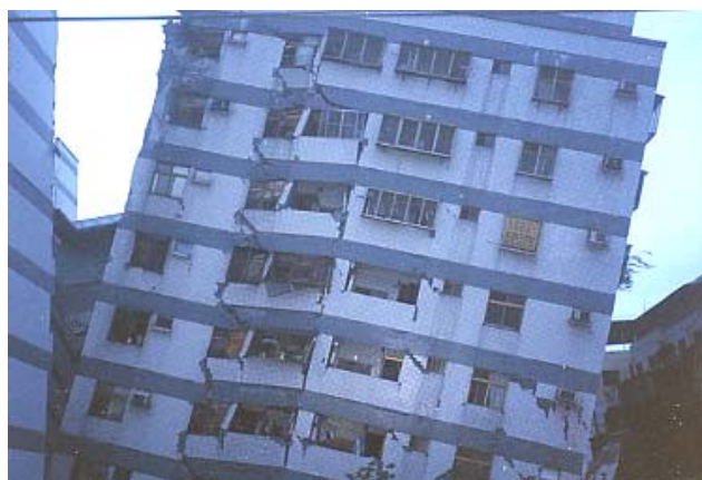
Figure 1-1 Undesirable (soft story) failure of RC SMF under Chi-Chi earthquake (1999)
