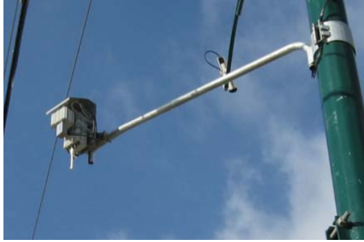
Figure 2-4 – Installed RSE Unit in USDOT POC Test Bed in Michigan
