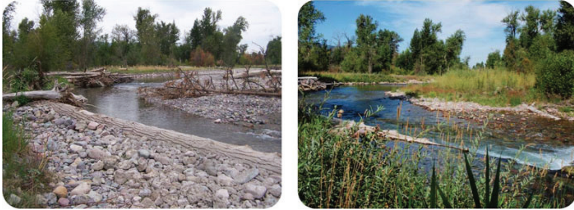
Fig 24: Log vein feature after installation (left) and at a later time (right)
