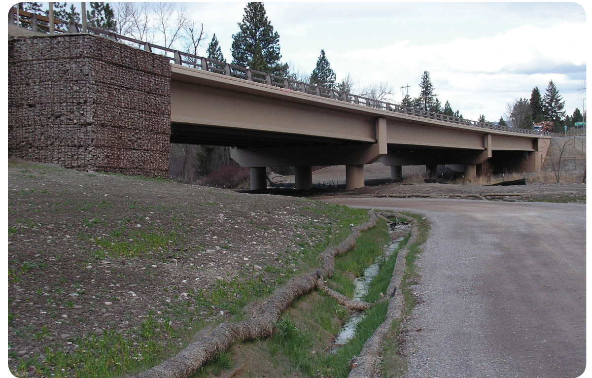
Fig. 2.1: The new Jocko River Bridge showing its multiple spans and the adjacent retaining wall. (photo credit: Brad Miller HDR Engineering)
