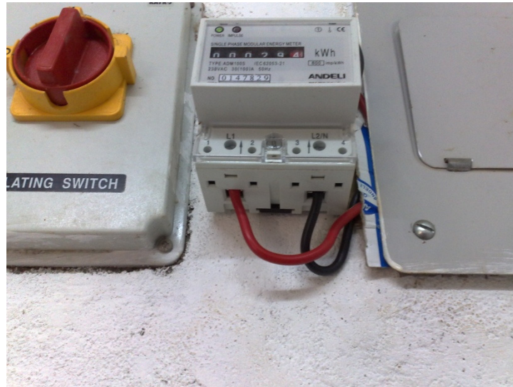
Image E-i 2: Analog electricity meter (Centre) connected to one of the buildings at Mpala
