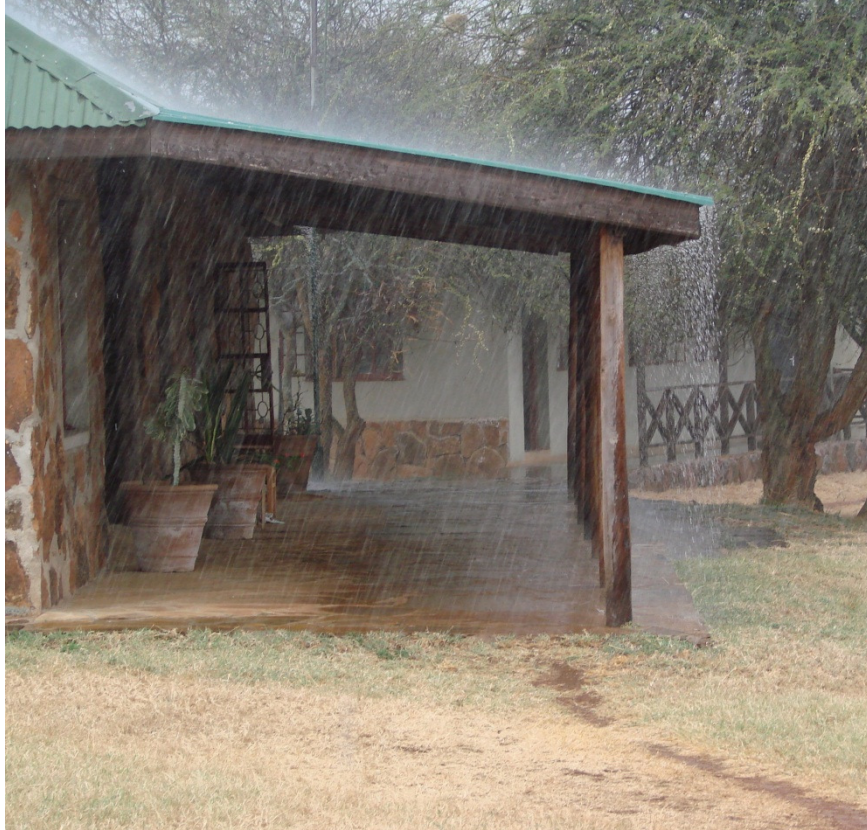
Image W-i 9: Administration Building during a rainstorm, showing lost run-off due to insufficient conveyance. Photograph by Ajay Varadharajan, 28 December 2010.
