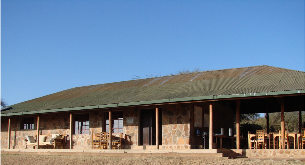
Image W-i 7: Mess Hall roof, showing degradation as a result of animal activity.
