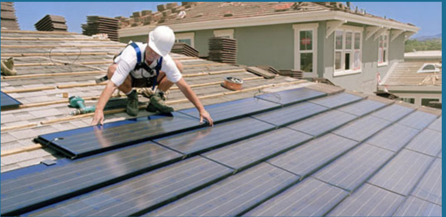
Figure 115: Renewable Energy Installation on a California rooftop
