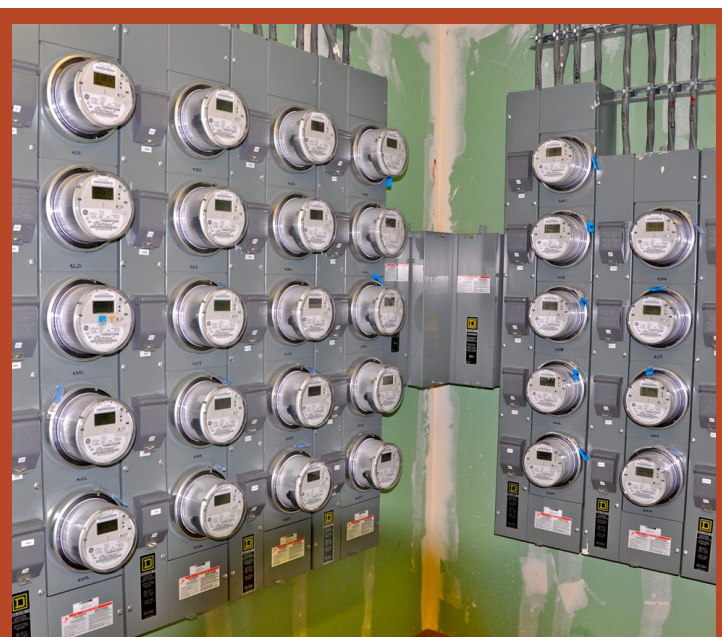
Figure 64: Pacific Gas & Electric Smart Meters
