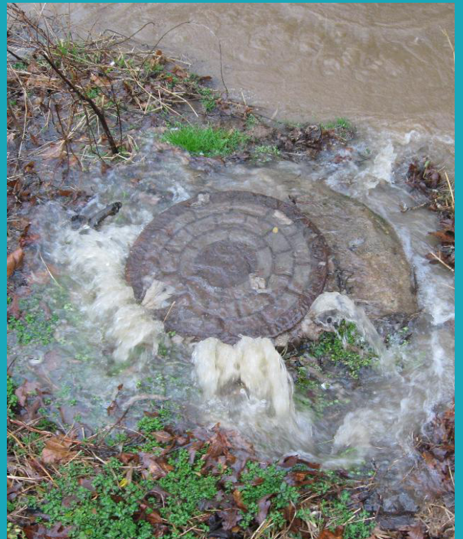
Figure 23: Storm sewer overflow
