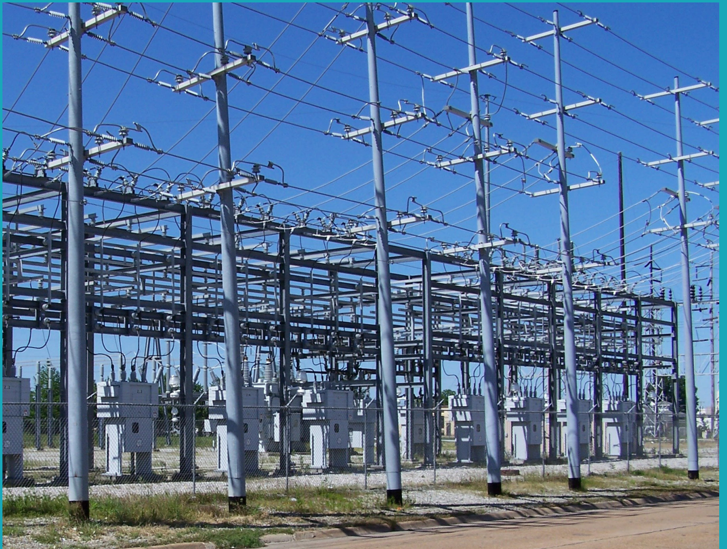
Figure 21: Sea level rise and increasing severe storm surges will threaten critical infrastructure such as the Gould Street Power Plant, which sits directly on the shoreline
