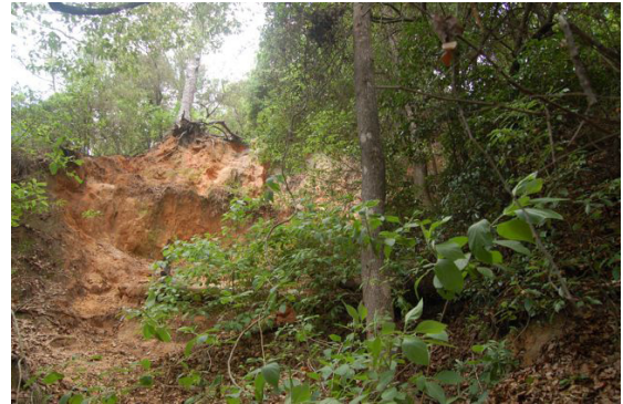
Figure 62- Erosion at Bay Bluffs
