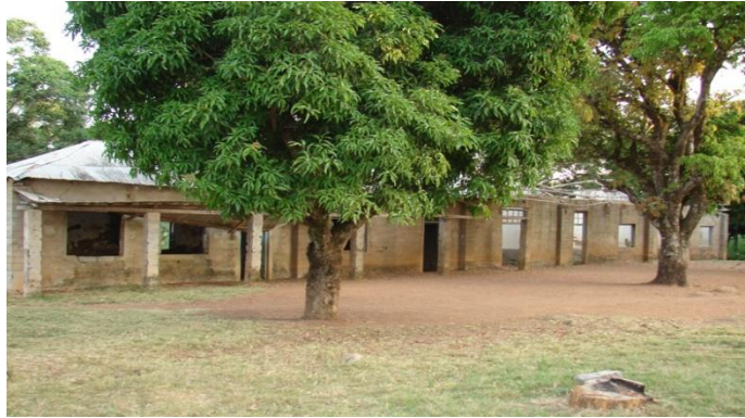
Figure 14: Dilapidated school building built in Ujamaa villages – Itira, Ukerewe - 2006
