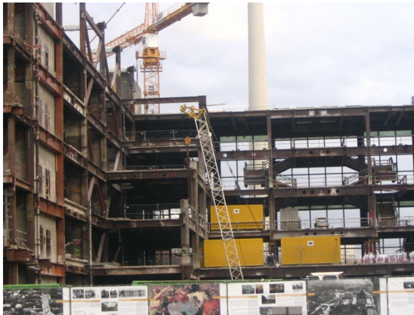
Fig. 33. Palace of the Republic demolition process, January 2007. Photo courtesy of Silke Atmaca.
