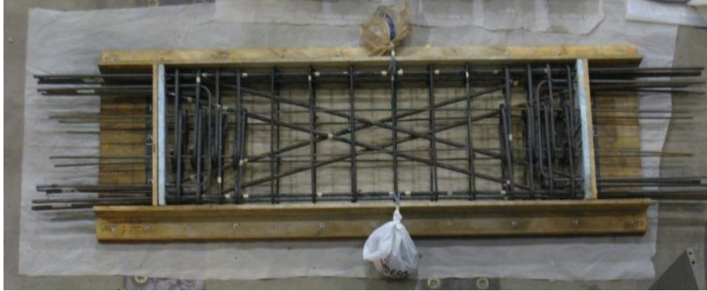
Figure 3.6 Coupling beam cage assembled in a wood formwork and ready for casting
