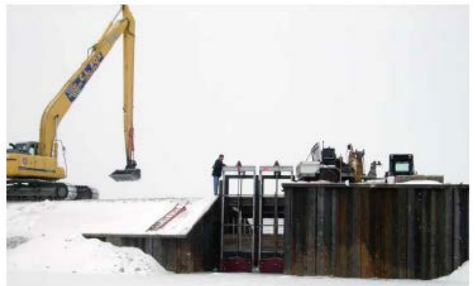
Figure 3.A.3: Construction of the water control structure on the diked wetlands at Crane Creek (DU 2011).
