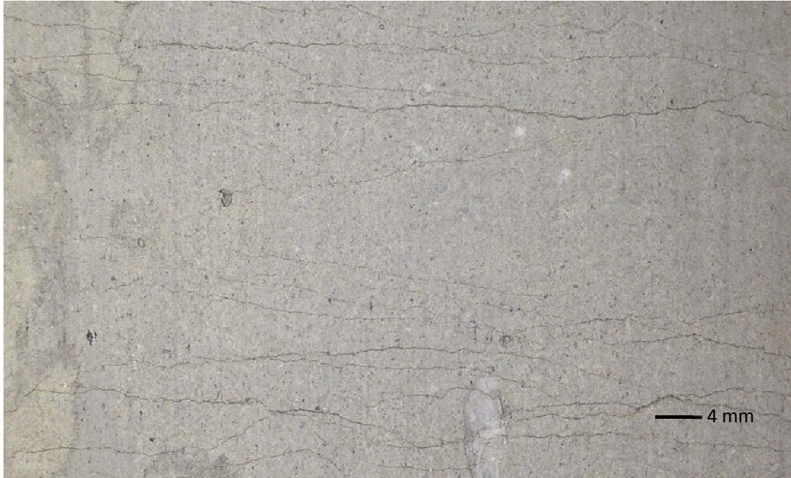
Figure 4-1, Figure of strained ECC specimen, showing multiple cracking
