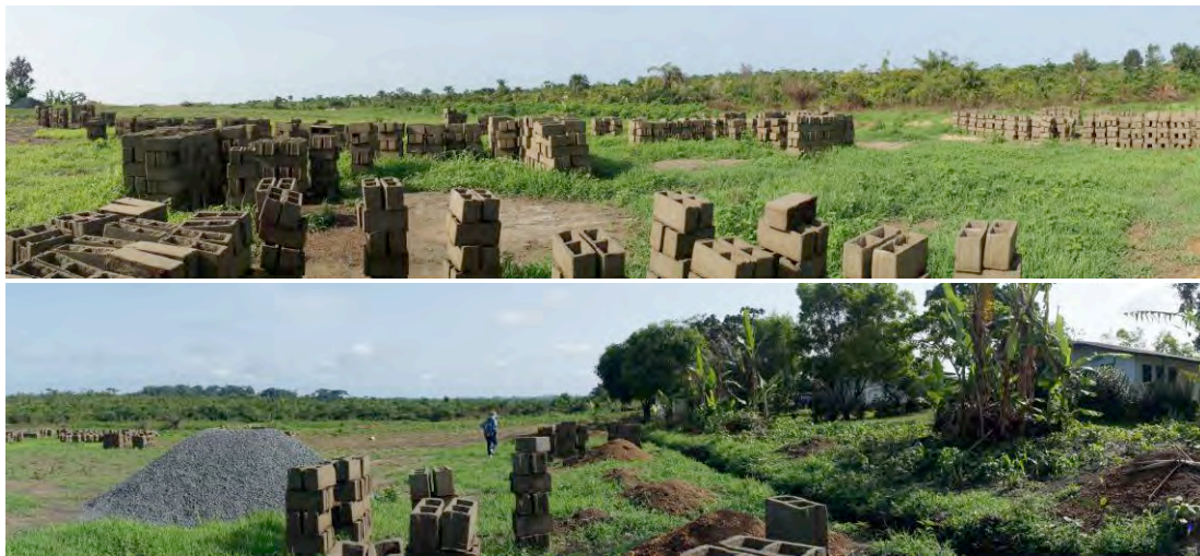
The site before construction looks natural and undisturbed, except some bushes were cleared from the site.
