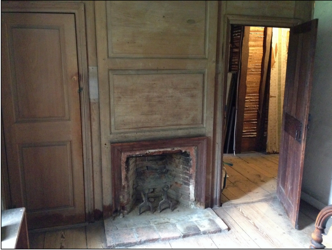
Figure 1.10. Fireplace and paneling in the Saint's Chamber, Old Manse. Trustees of the Reservation
