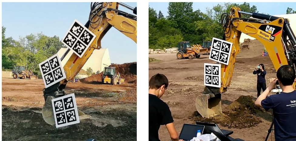
Figure 2.20 Bucket linkage generalized mapping prototype installed on backhoe
