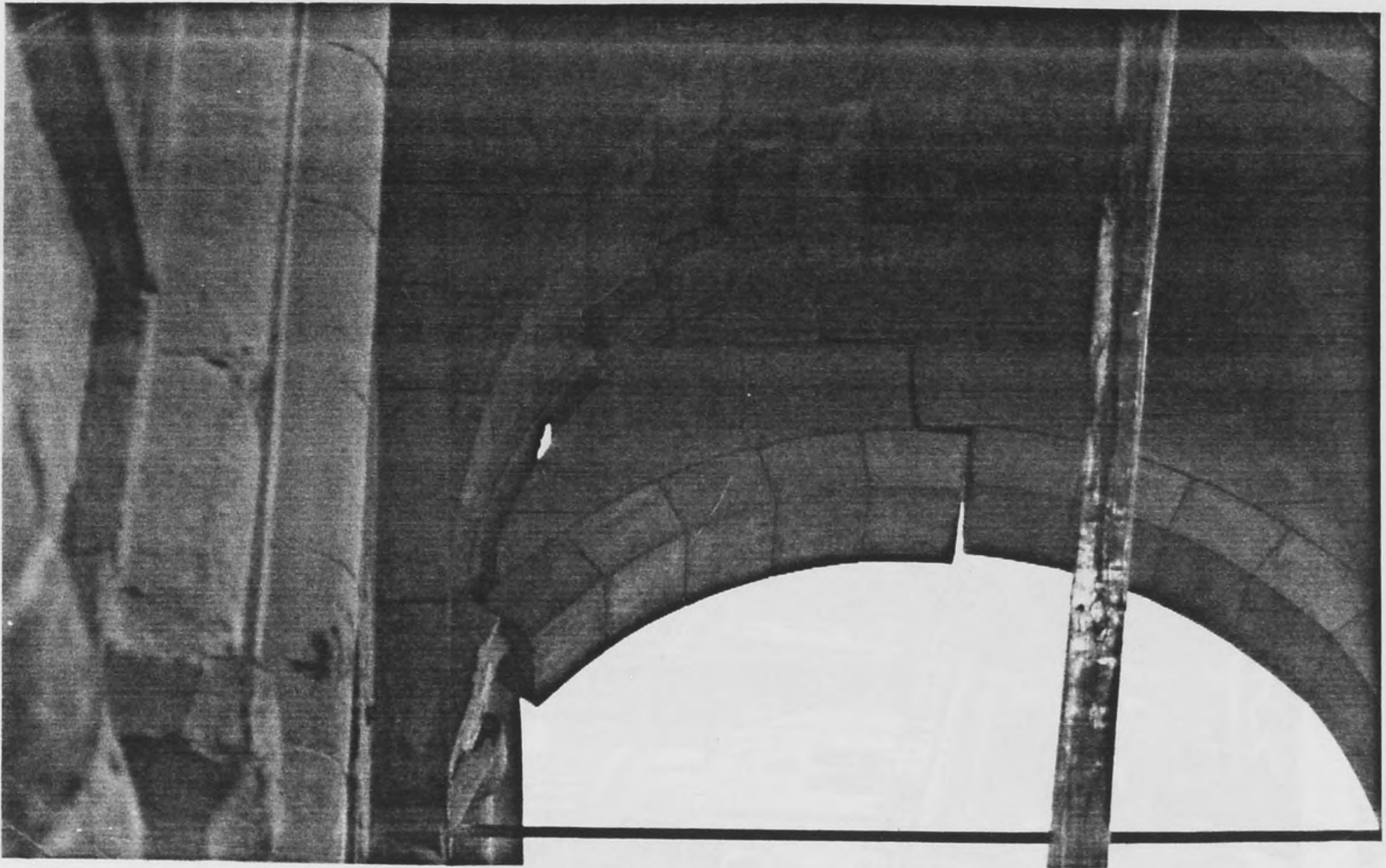
(b) Loose stones in arch
