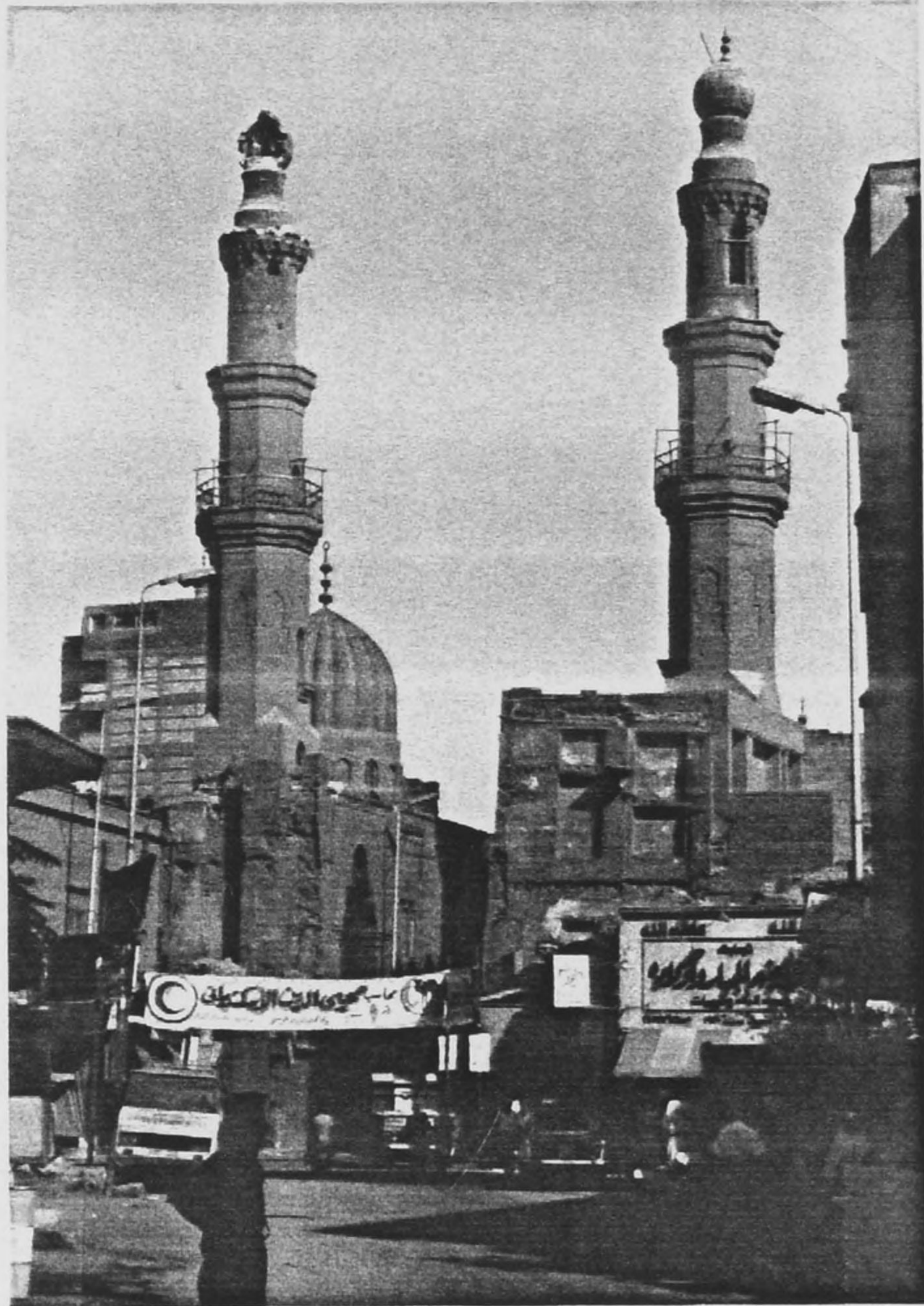
Fig. 25 Partially collapsed top of minaret at Amir Shaykhu Mosque
