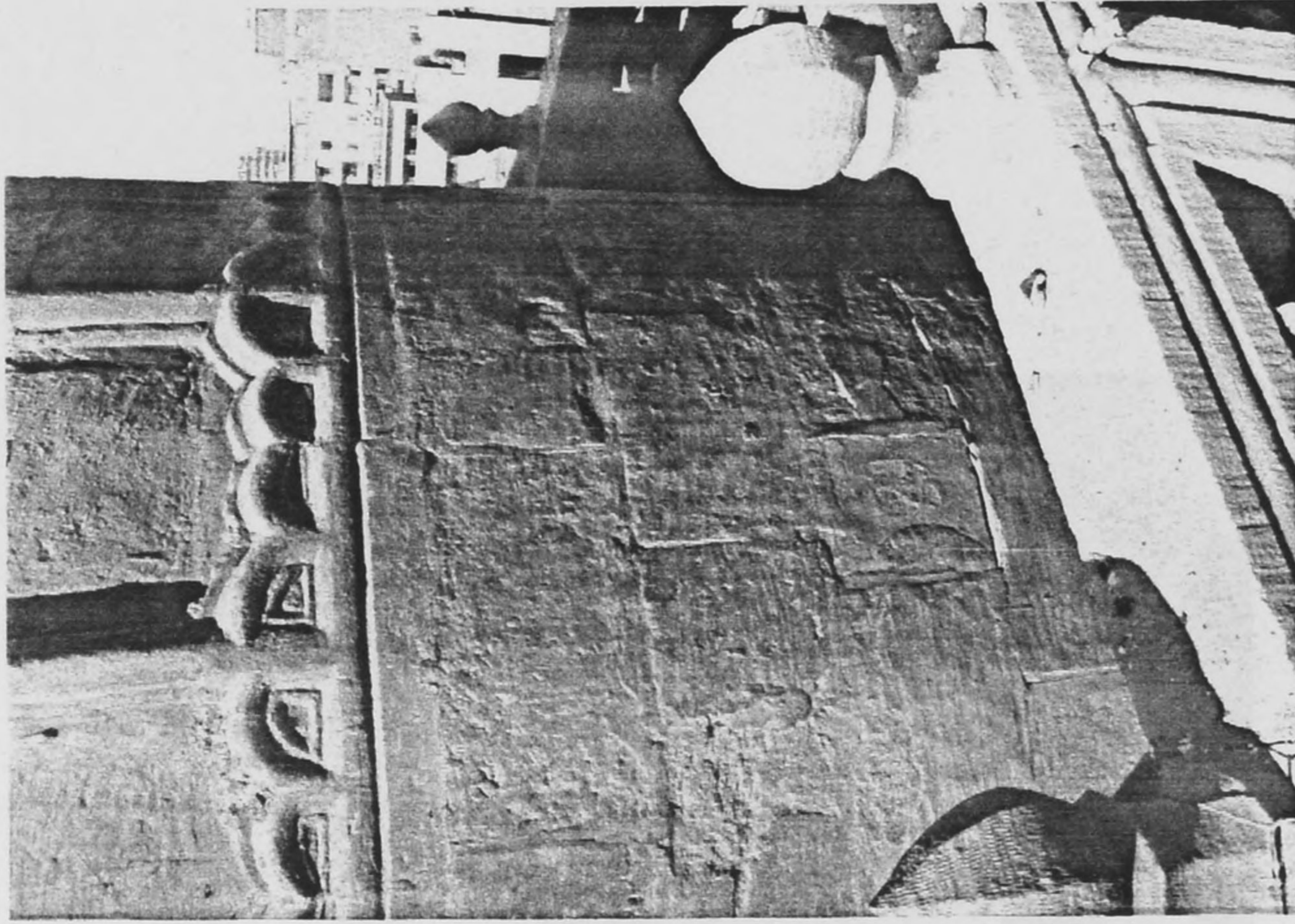
Fig. 24 Cracking and spalling along cracks in minaret tower section above roof of mosque
