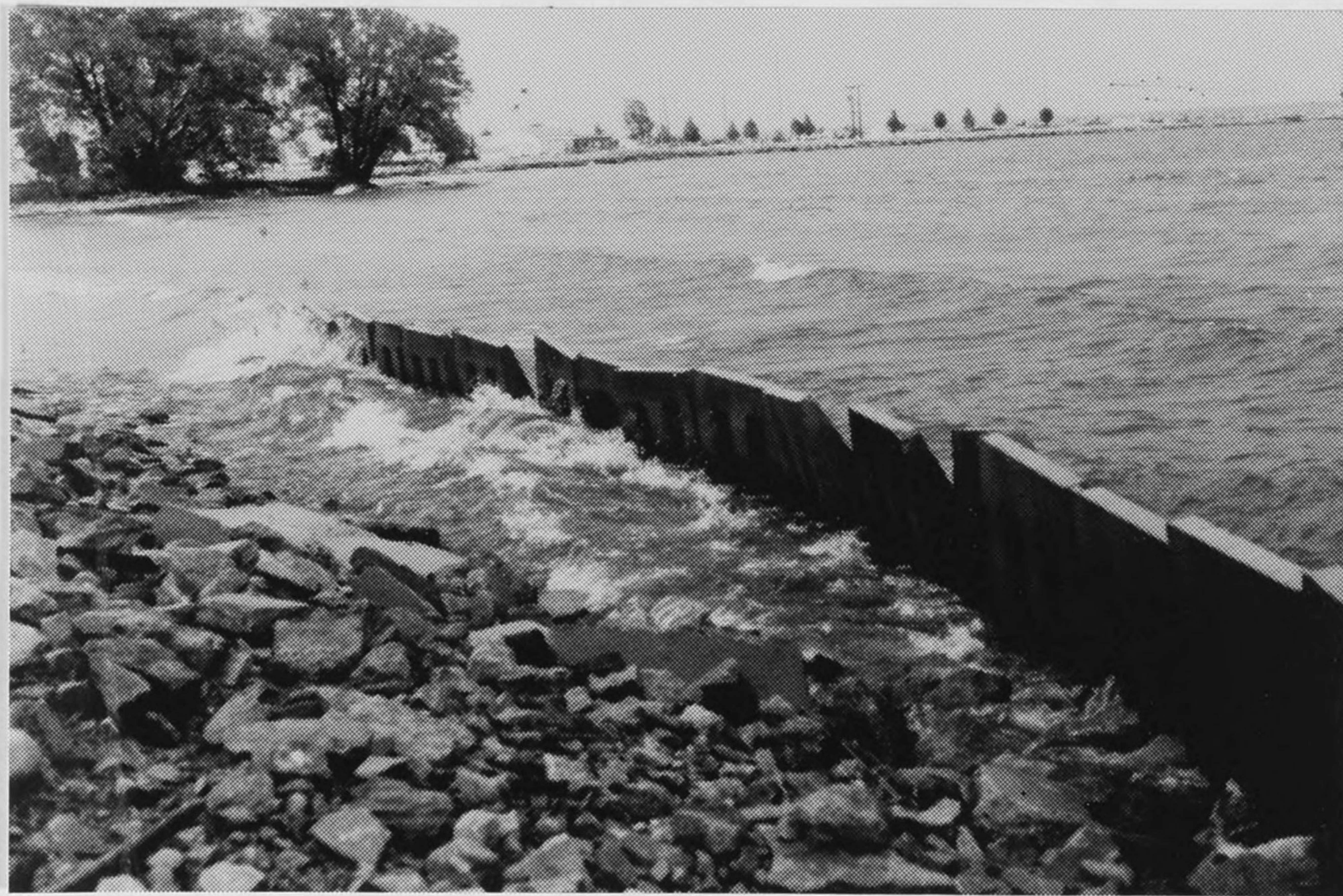
Figure B60. Site X: Normandy type wavebusters in front of 240 S. State. Note revetment almost immediately behind wavebusters.
