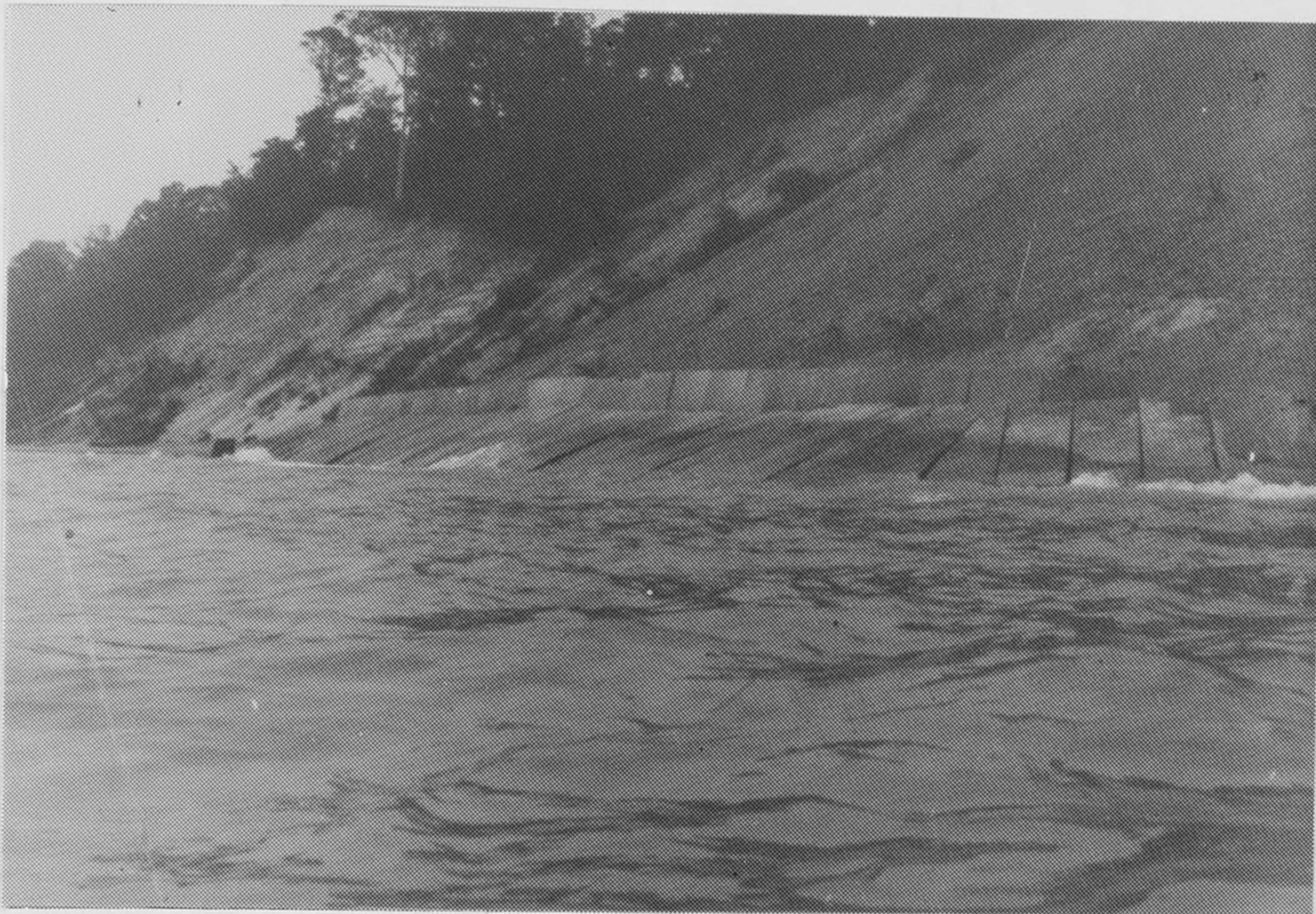
Figure B7. Site C: View of modular units looking from offshore onto the structure.
