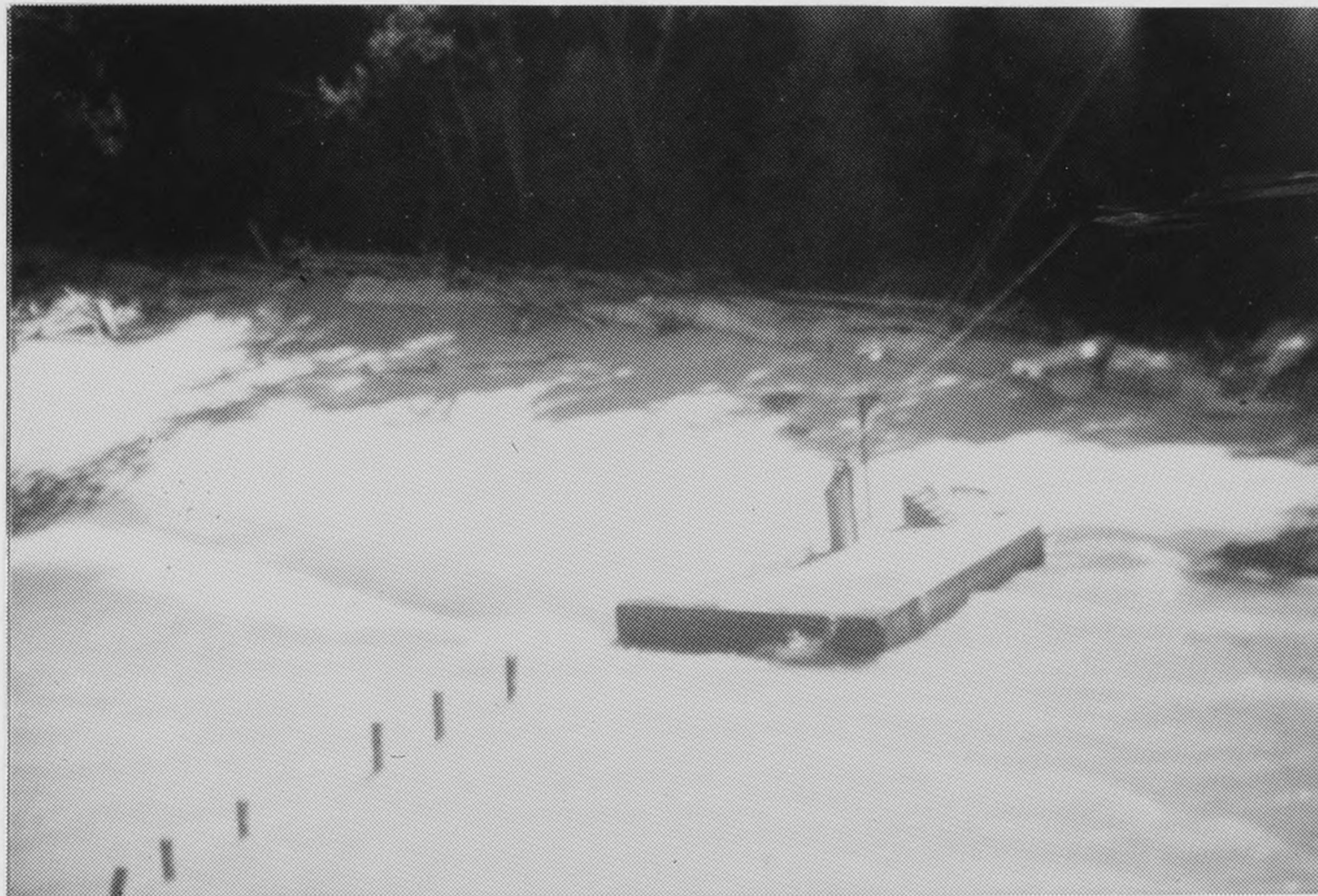
Figure B4. Site B: Aerial photograph of concrete foundation block for tramway, at southern edge of property. The shoreline is at the outside edge of block on the north side and at the landward edge to the south.
