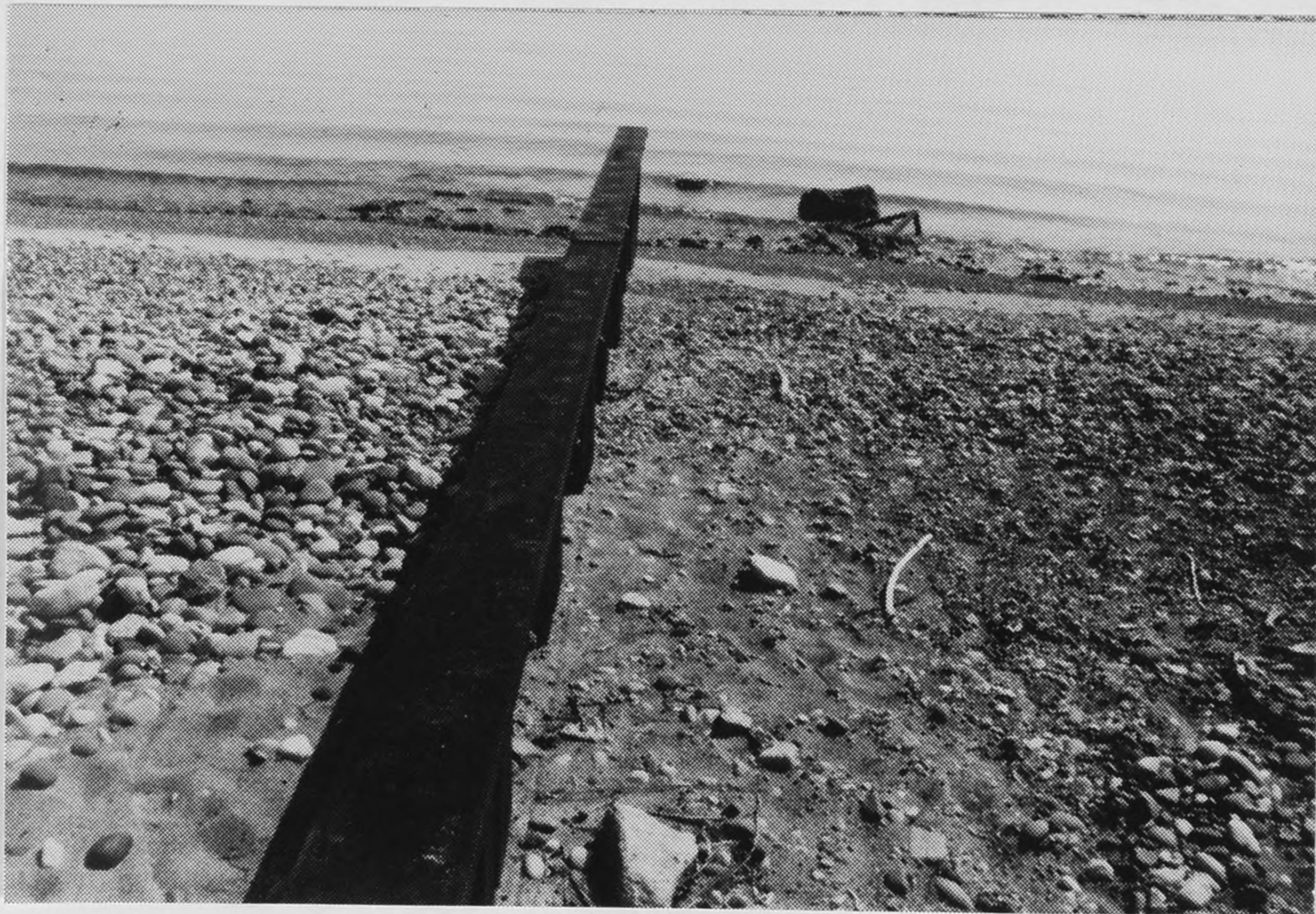
Figure B76. Site II: Looking offshore along most southern groin. Littoral drift is left to right. Note coarse cobble on updrift side of groin.
