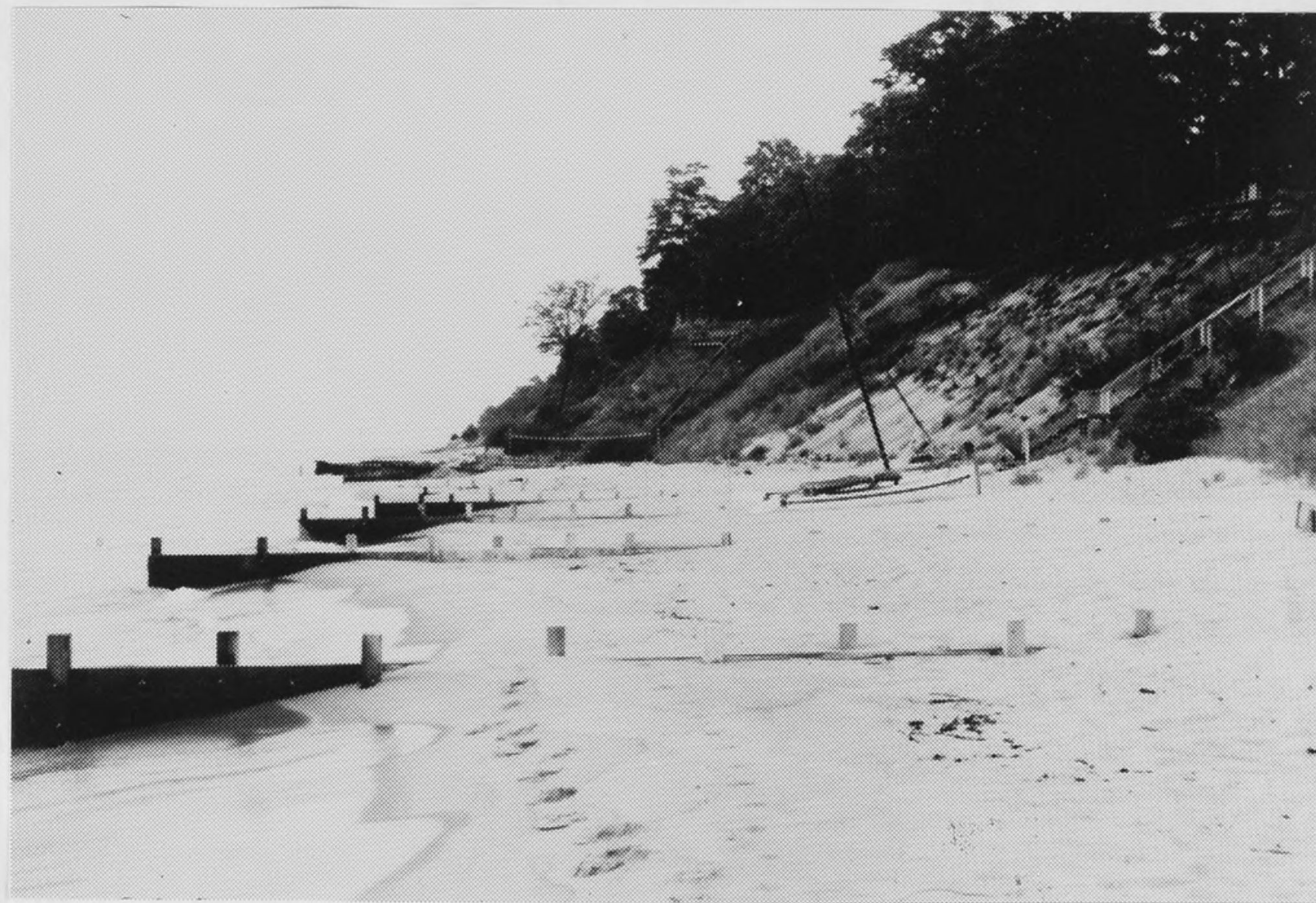
Figure B15. Site F: Looking north towards the site. Buried groin is to the north of the four groins in the foreground. Note longer and higher groins on either side of property.
