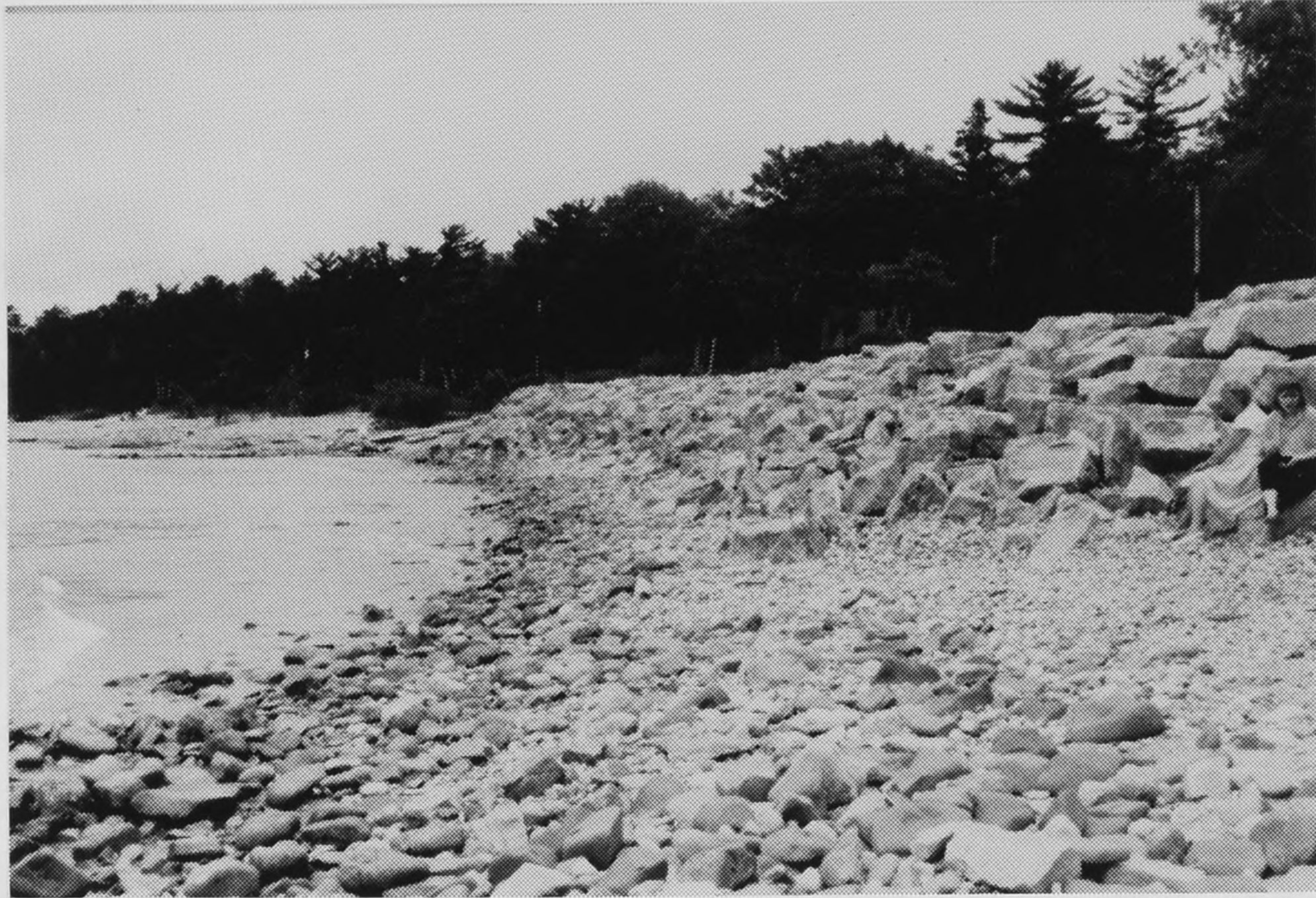
Figure B59. Site W: Looking at coarse beach in front of revetment.
