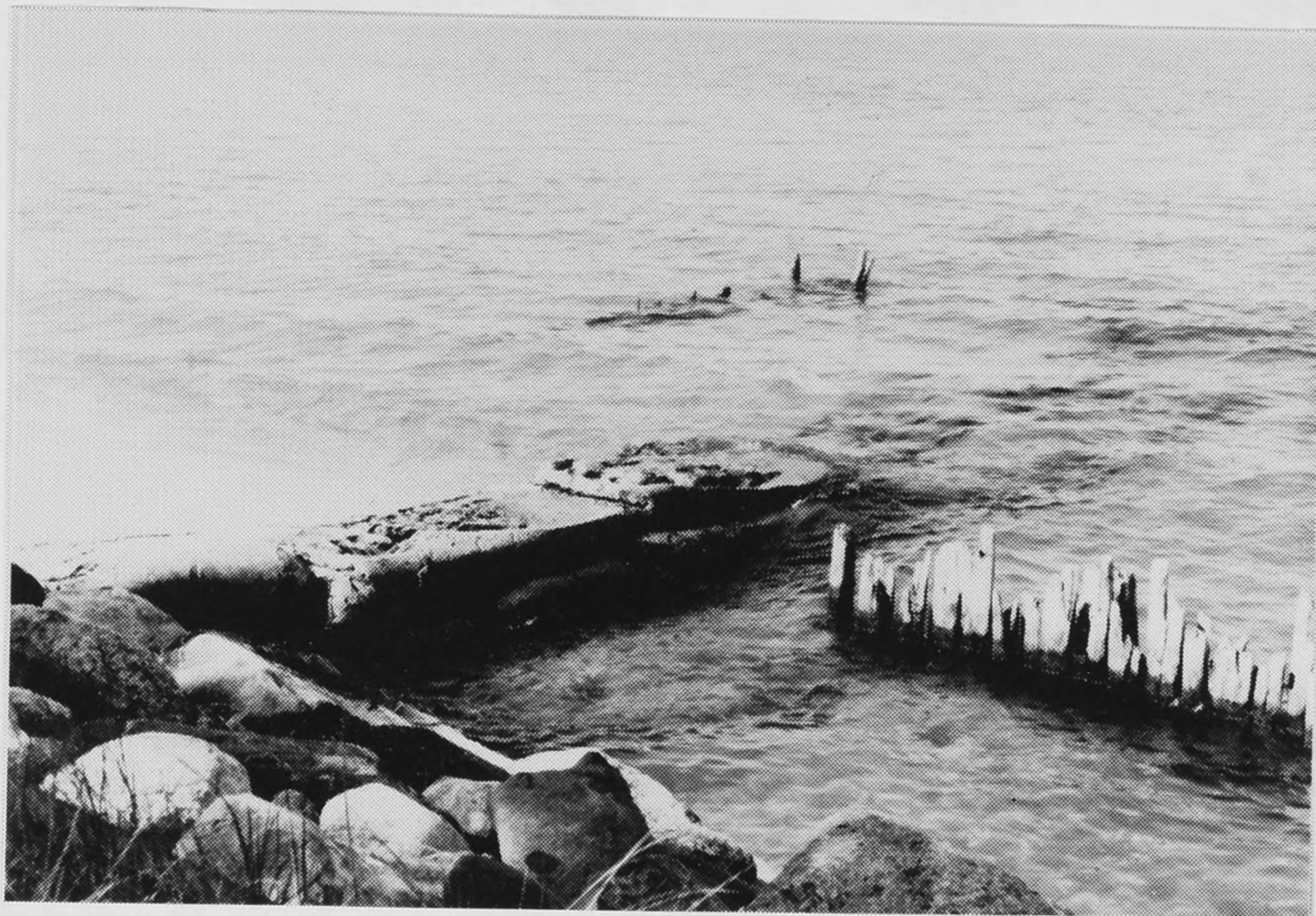
Figure B25. Site J. Tube groin just to north of one in Fig. B24. Note damage to groin top and sand accumulation on south side.
