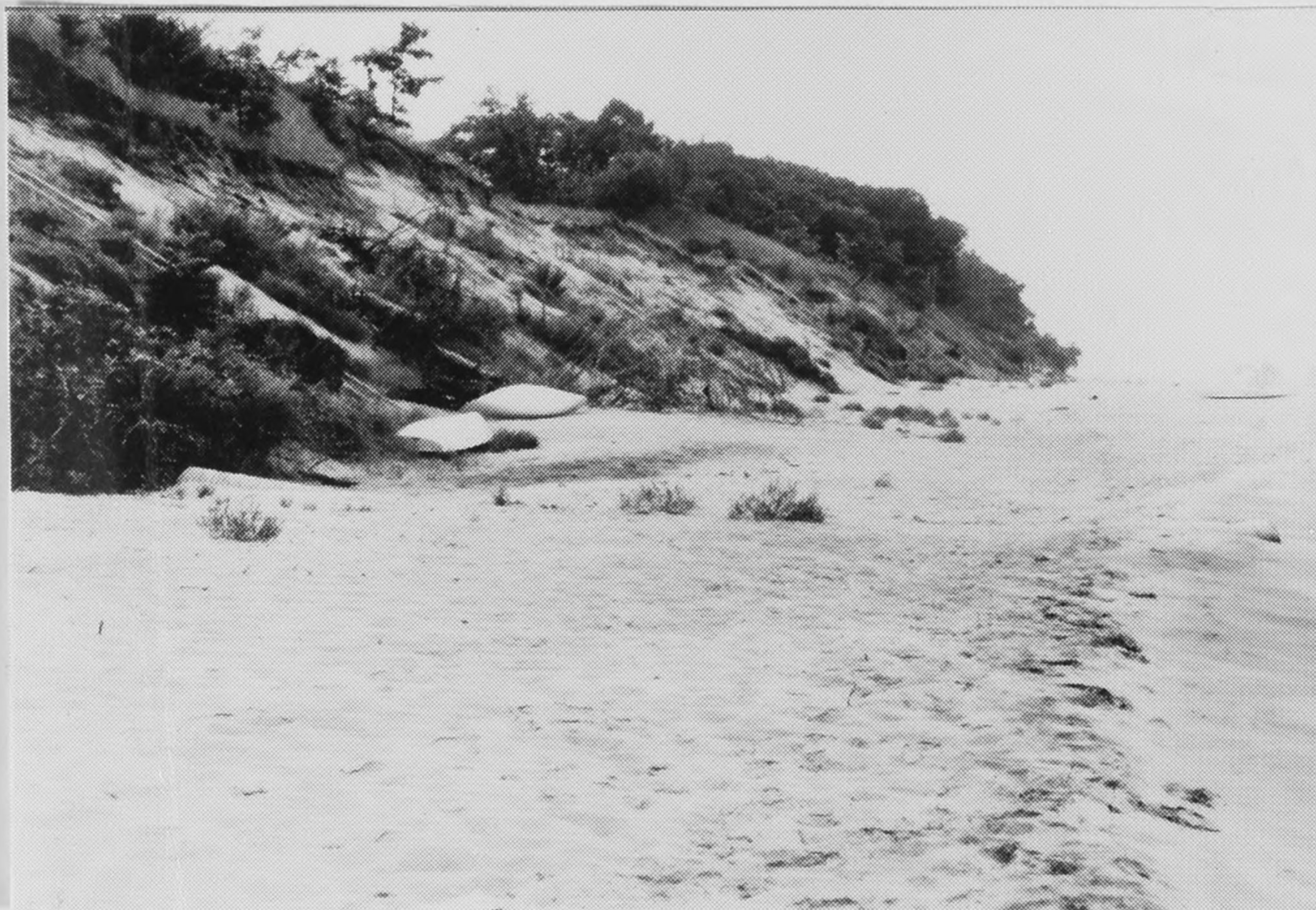
Figure B16. Site G: Looking directly onshore from beyond end of groin, Note that groin is almost completely buried with no beach elevation difference across groin.
