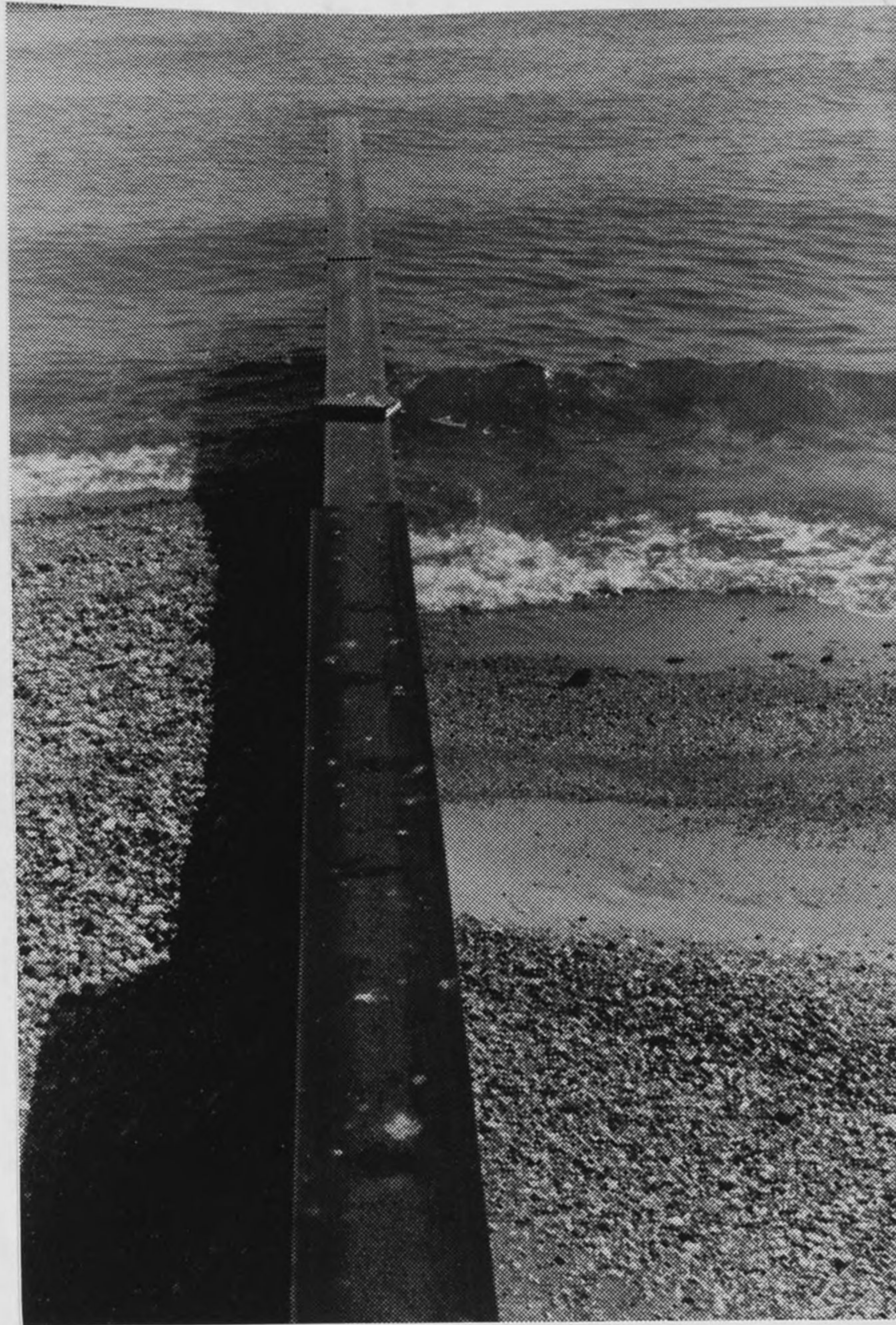
Figure B72. Site GG: Looking offshore along Durand groin. Littoral drift is left to right.
