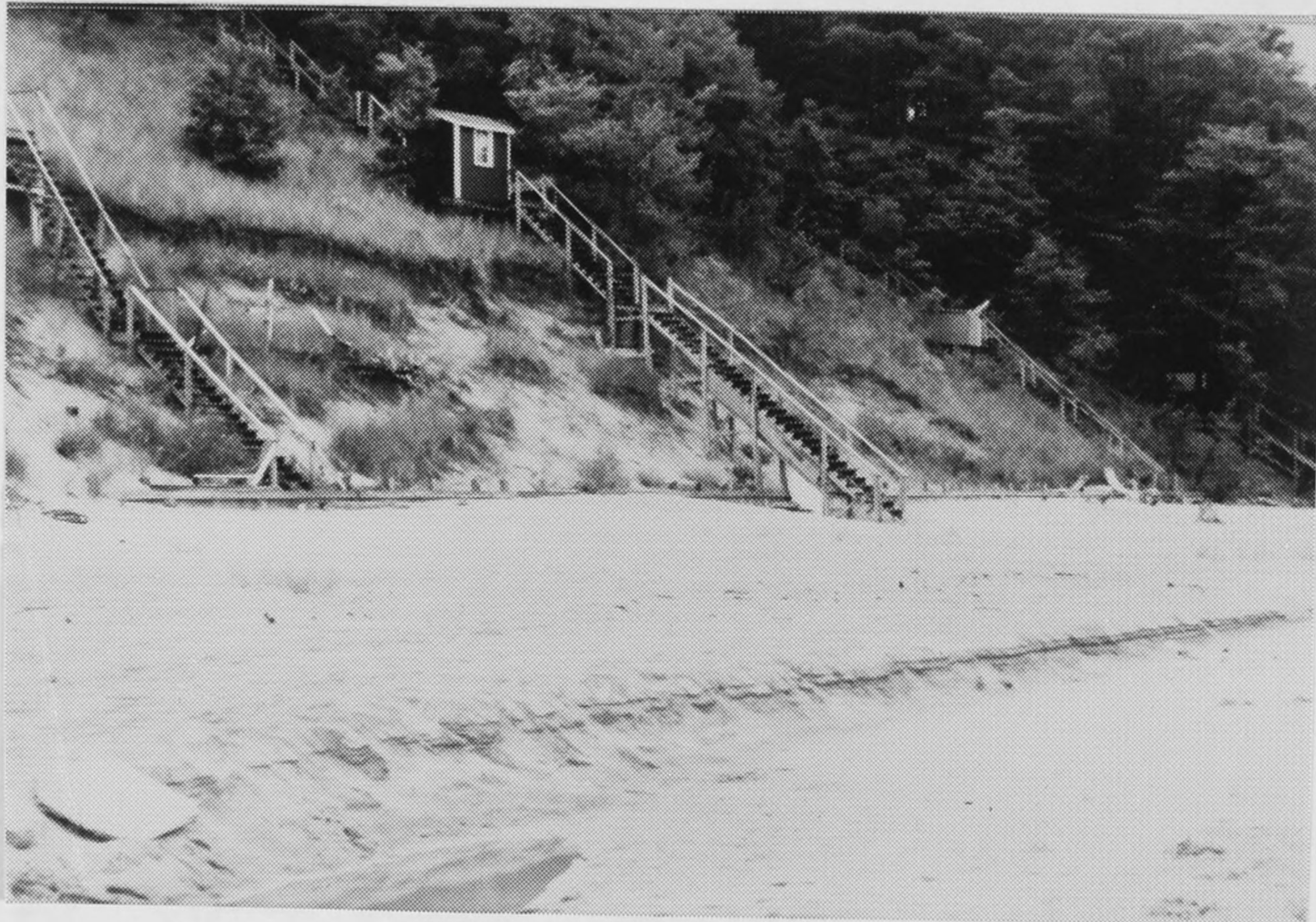
Figure B11. Site E: Top of retaining wall is visible at toe of bluff. Straight line in foreground is where beach level drops immediately at shoreline with beach perched more than 12 inches above water level. View is towards south.
