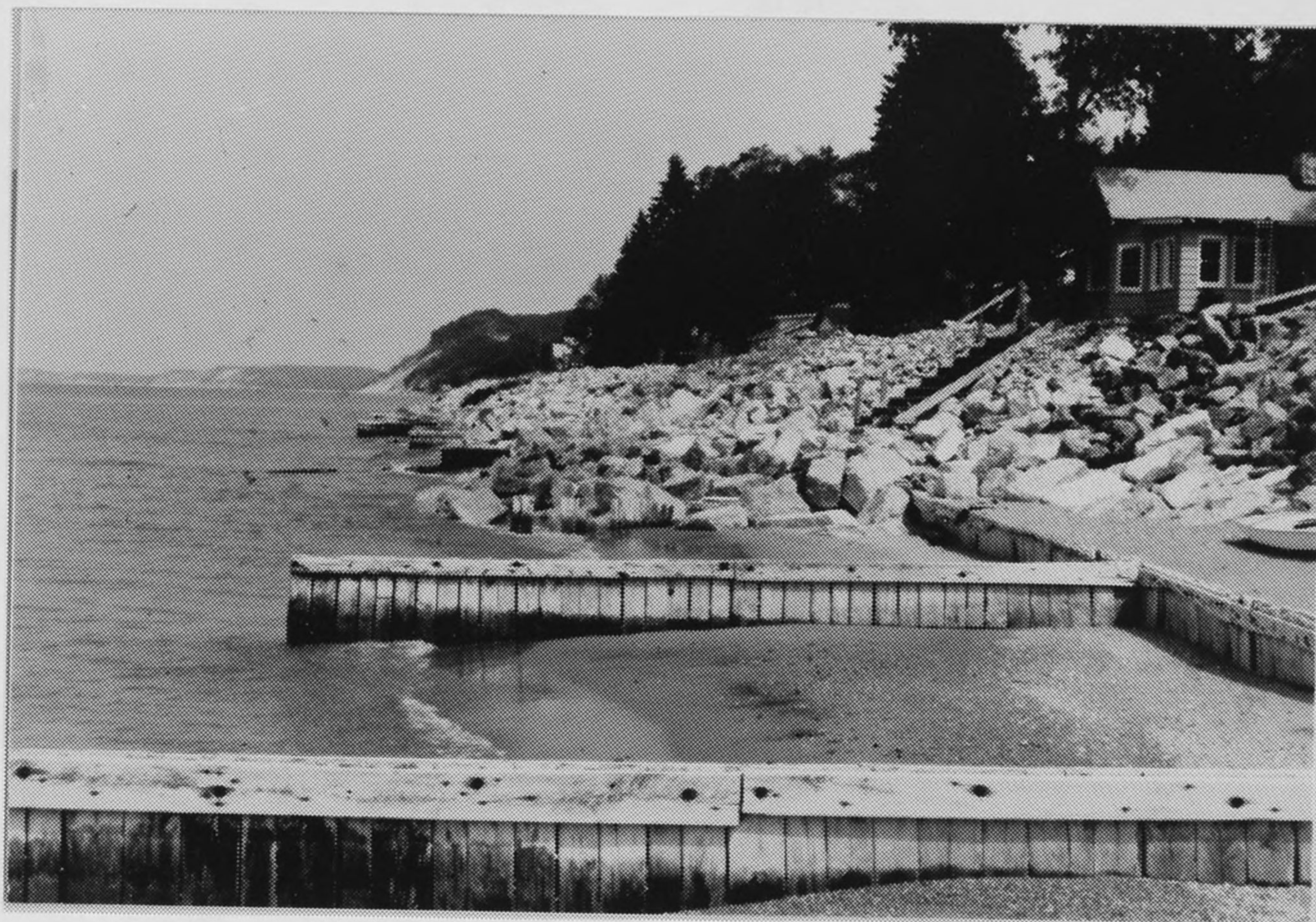
Figure B40. Site N and O: Looking north towards the long revetment on site O from Site M and N property. Revetment on site N is just visible to the right and well up above the existing water level. Also groin and sill system exists between revetment and shoreline. Note old groins within revetment on site O.
