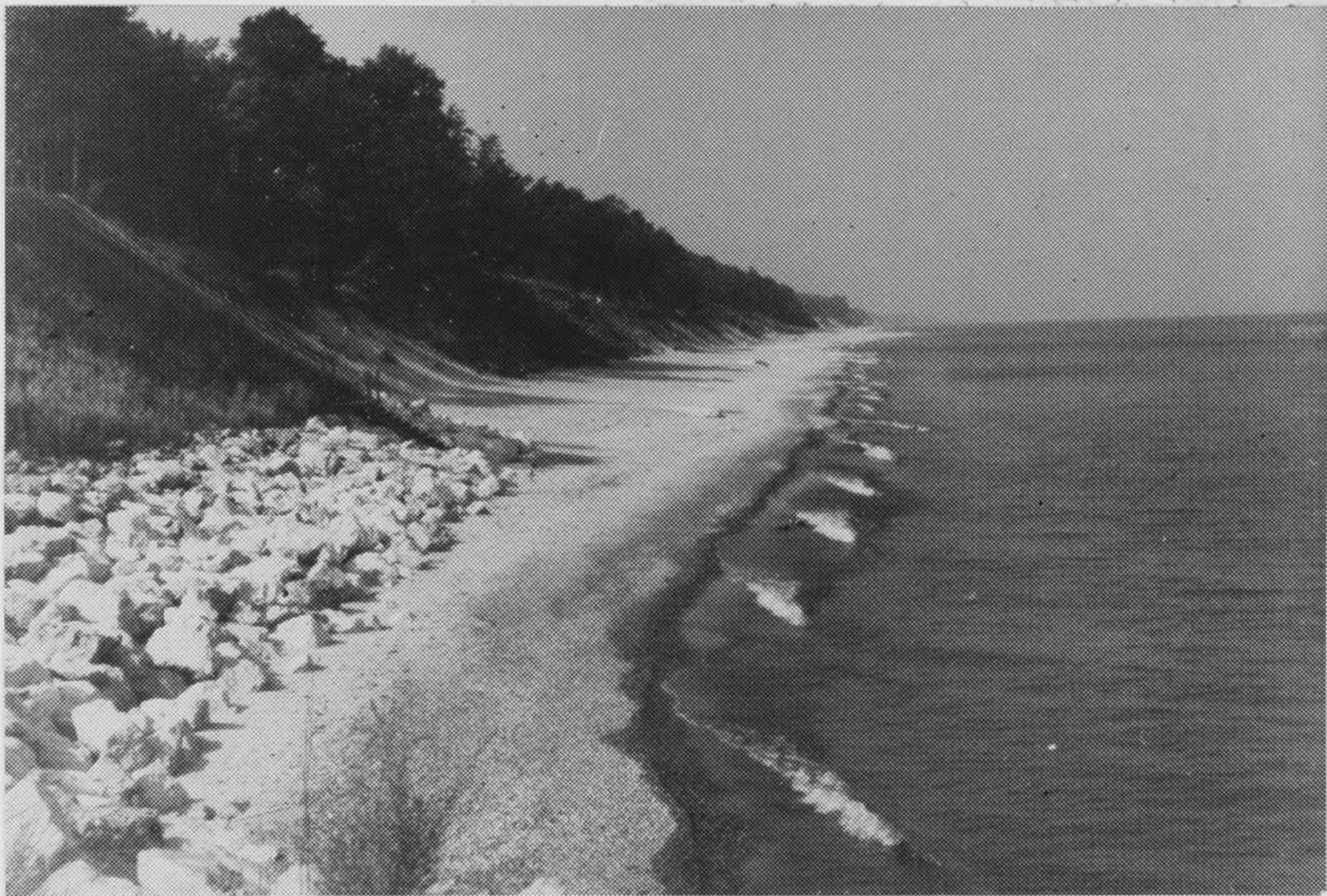
Figure B2. Site A: Looking along beach in a southerly direction from revetment just north of property. What appears to be groin ends is actually the end of the second tier of bags and groins extend into the water.
