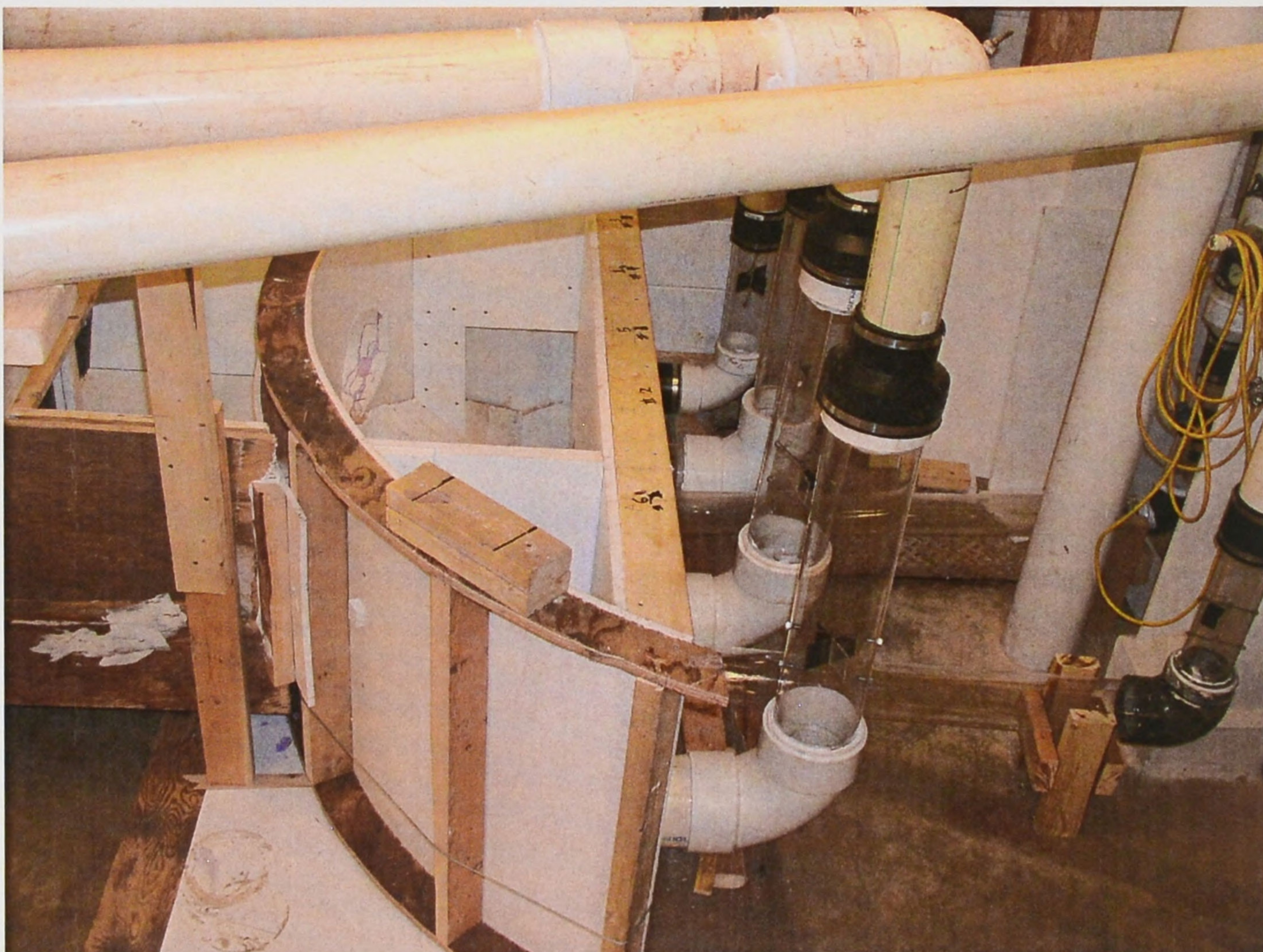
Figure 5. Wet Well and Pump Intakes.
