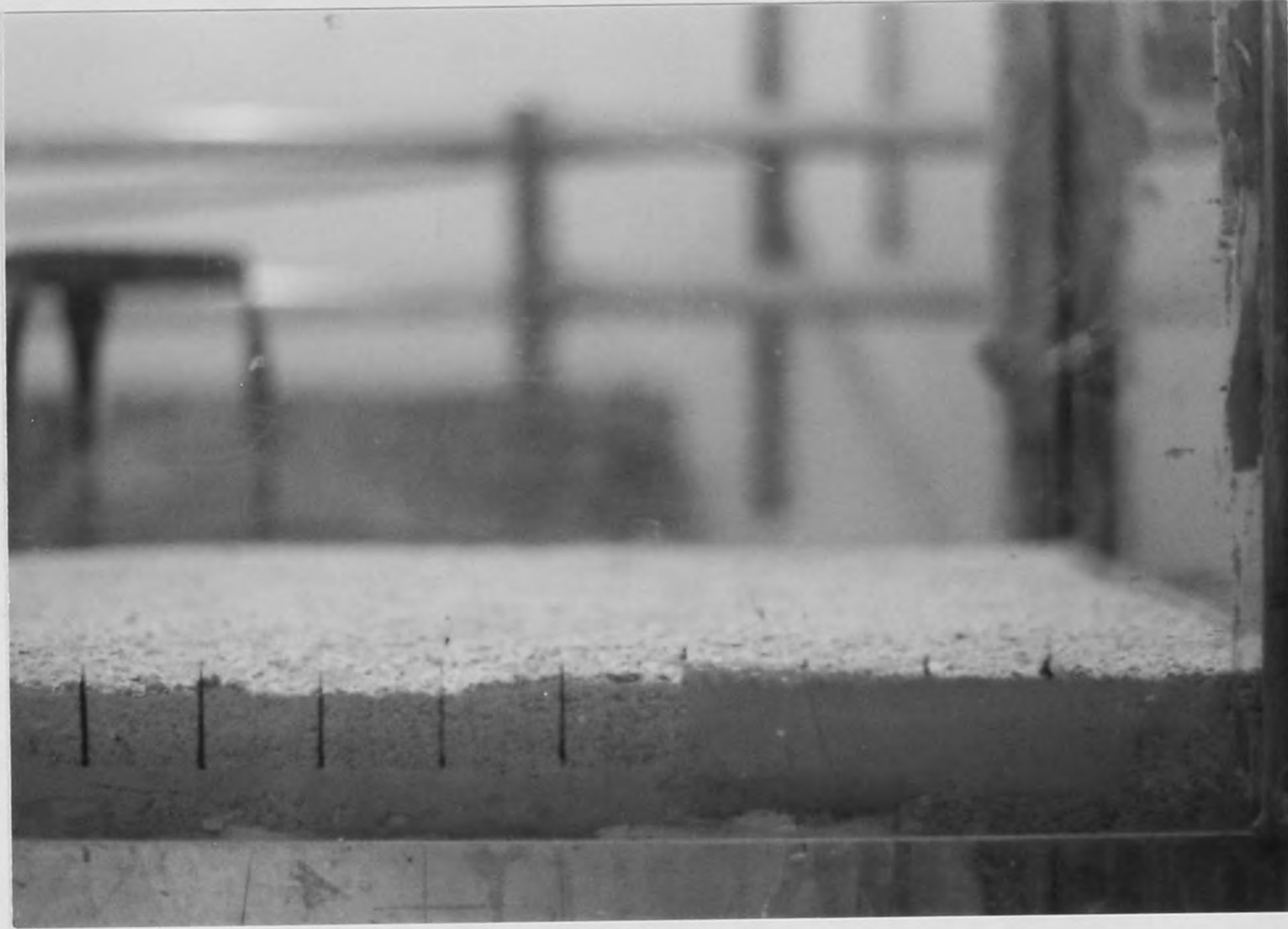
FIG. 2. Preliminary Stage of Test Section Construction (Placement of 3.5 inches of the Sand Isolation Layer)
