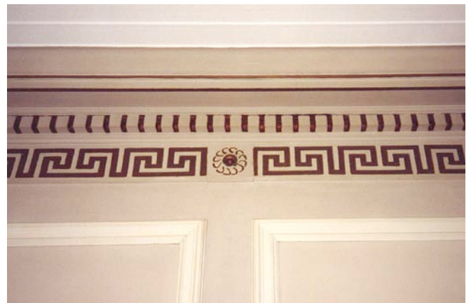
Crown molding detail in dining room (Note gold Greek crosses that were too expensive to repaint in renovation)
