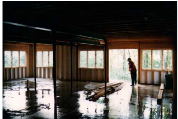
And the basement floods
