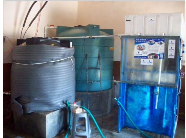
Nawalgarh: RO and water treatment unit
