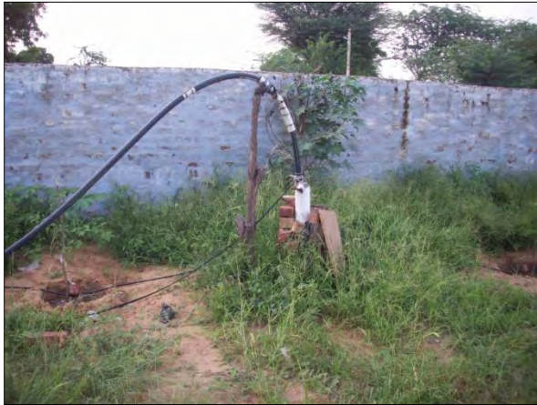
Taranagar: Source water borewell
