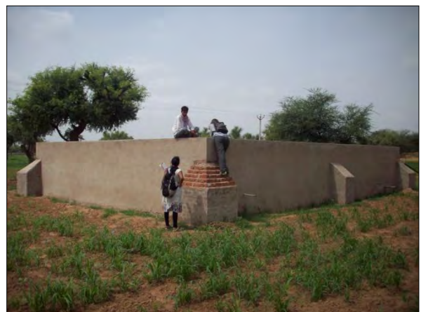
Mukundgarh: RO brine storage basin
