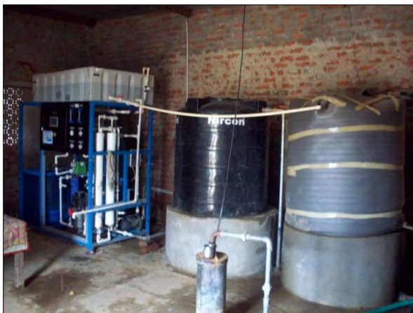
Sitapura: RO and water treatment unit
