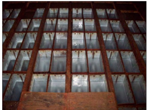
Ice Factory (Mukundgarh): Cooling tank (07/20/11)
