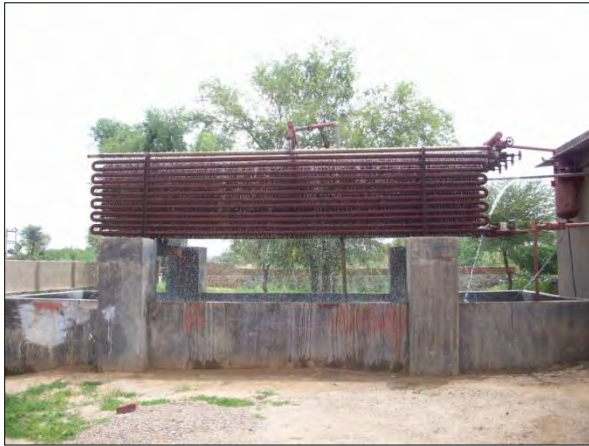
Ice Factory (Mukundgarh): Cooling pipes (07/20/11)
