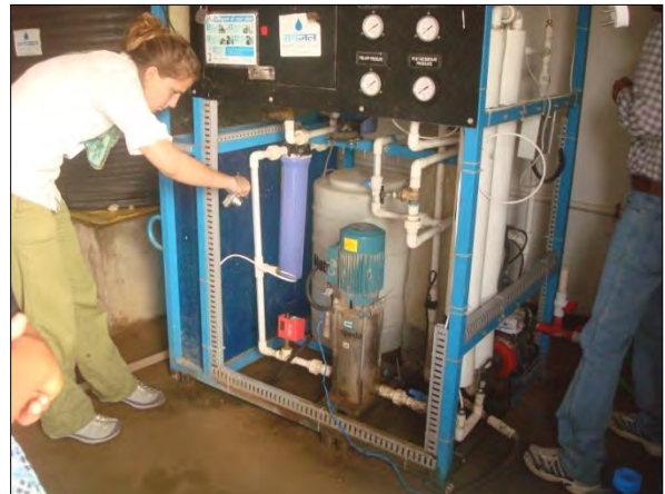
Mandawa-2: RO and water treatment unit
