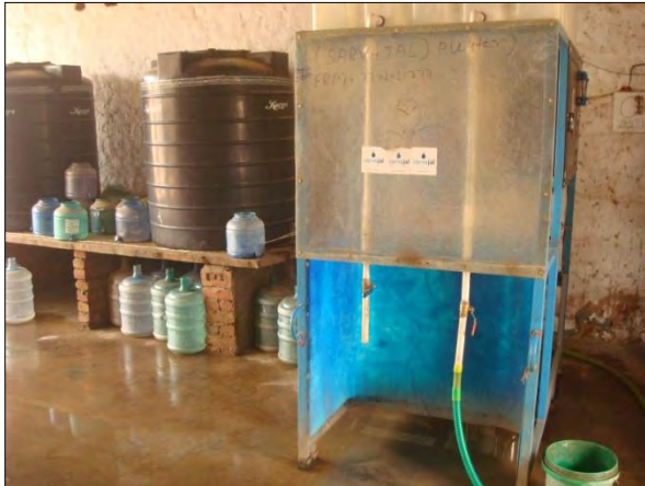
Ramgarh-1: RO and water treatment unit (back)
