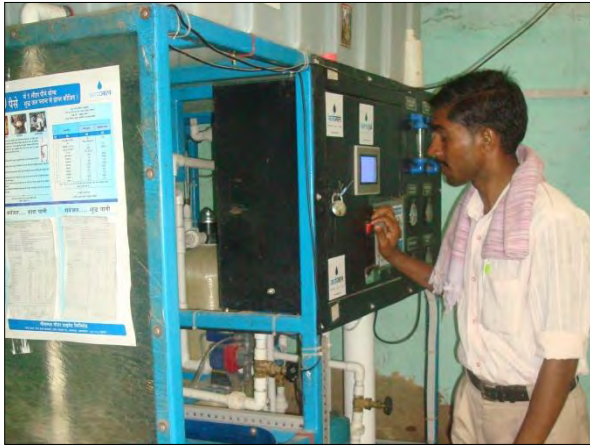
Fatehpur-2: RO and water treatment unit
