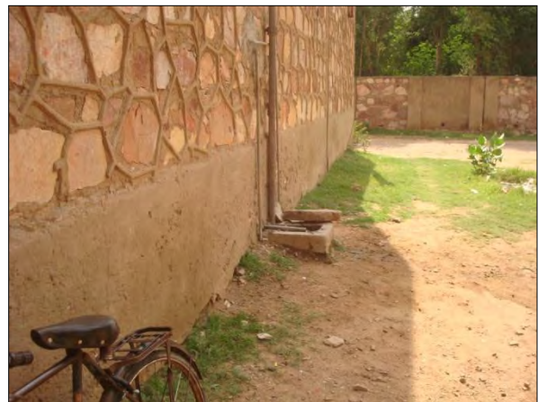
Copper-1: RO brine discharge on side of building
