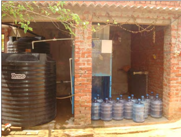
Gothara: RO unit and operations building
