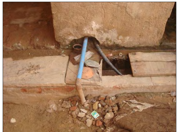
Mandrela: RO brine discharge to sewer
