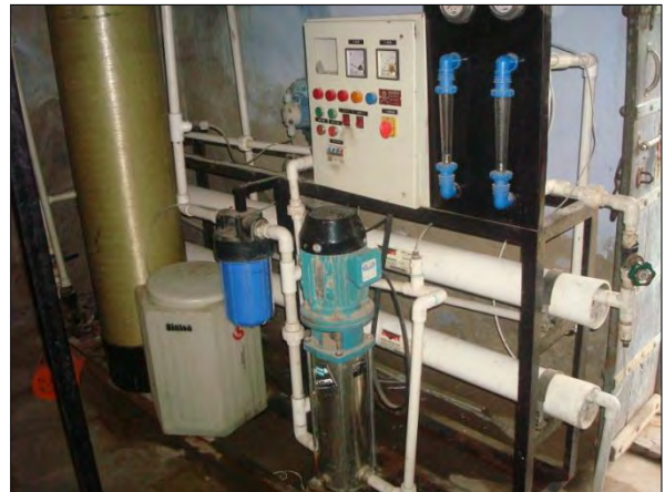
COCO (Bagar): RO and water treatment unit
