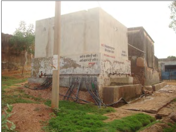
Choti Pancheri: RO unit and operations building
