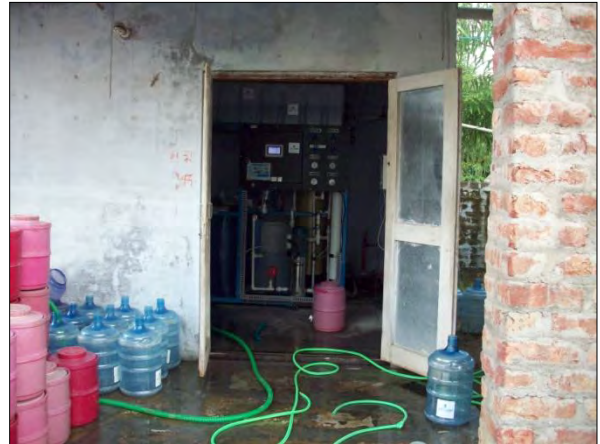
Taranagar: RO and water treatment unit
