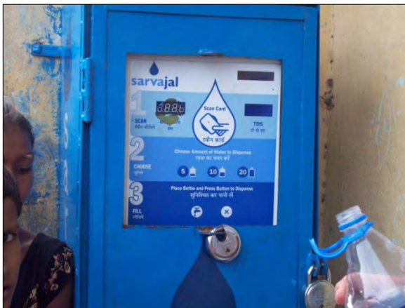
Tekra Slum: Water ATM pilot installation in Tekra, a slum in Ahmedabad (07/12/11)
