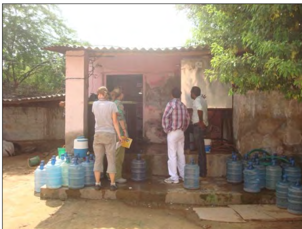
Malsisar: RO unit and operations building
