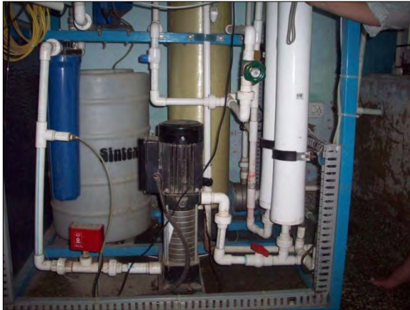
Headquarters: RO and water treatment unit in Ahmedabad (07/12/11)
