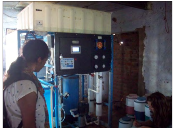
Mukundgarh: RO and water treatment unit
