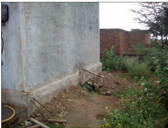
Rajgarh: RO brine discharge on side of building
