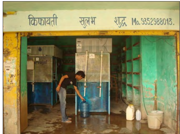
Copper-1: RO and water treatment unit
