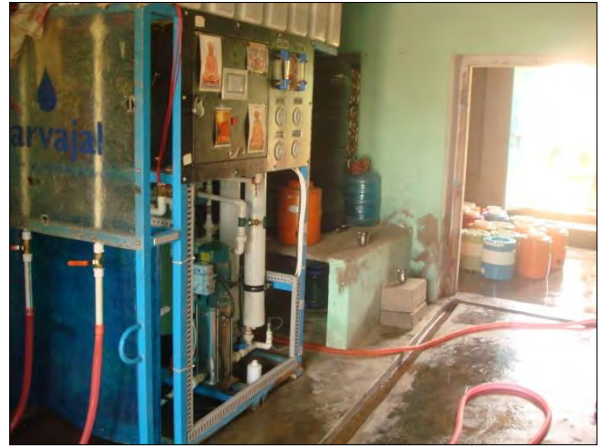
Bissau-2: RO and water treatment unit
