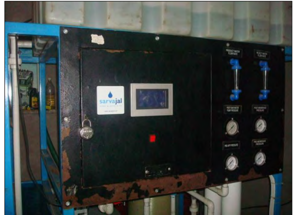
Siriyasar Kalan: RO and water treatment unit
