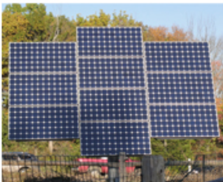
School 3: Sun-seeking solar panel moves with sunlight to maximize solar intake.
