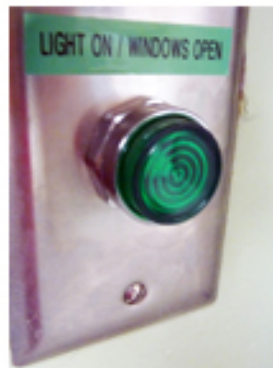
School 3: Green light helps occupants know when to open windows.
