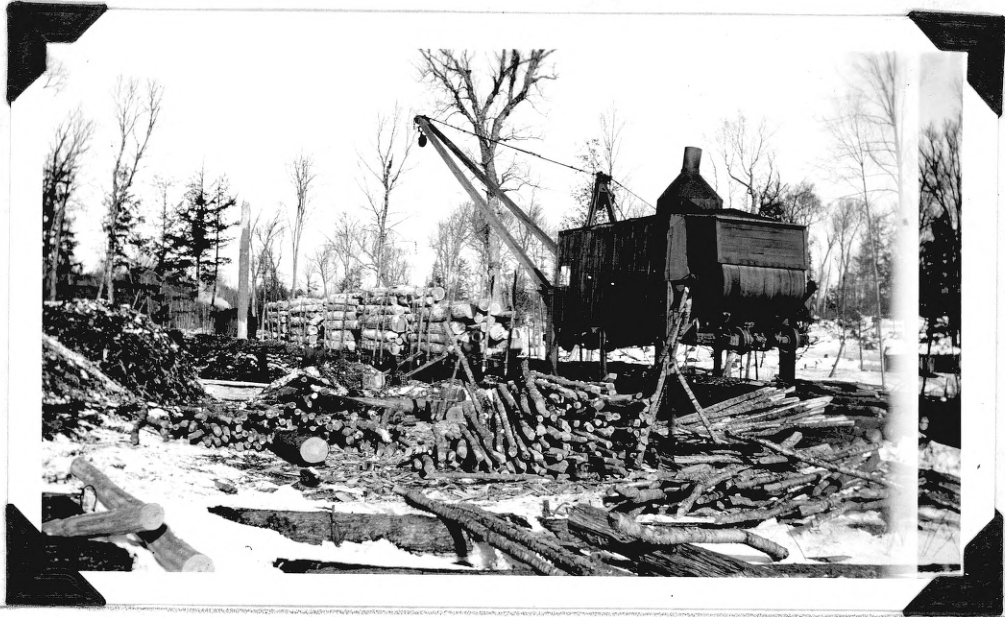
McGifford loader in action. Note car stakes piled in foreground of picture. Their use depletes growing stock of forest and is an expensive item in operations.
