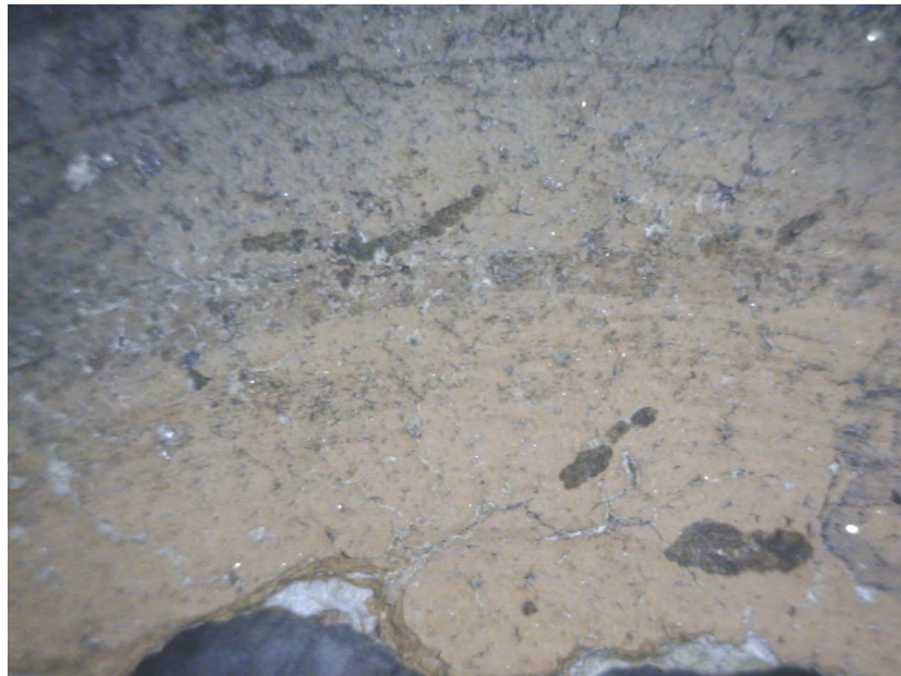
Figure 27. Interior cracking at 20x magnification (MUS 2347)
