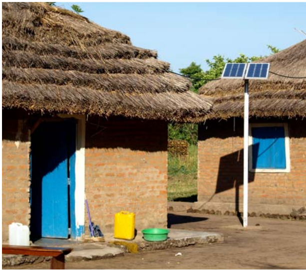
Figure 2. Solar Home System
