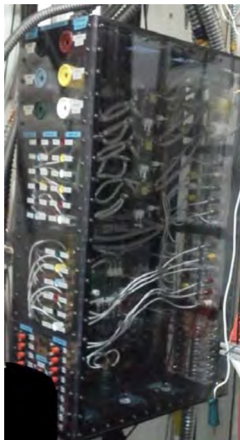
Figure 4.16. X3 NHT power and telemetry breakout box.
