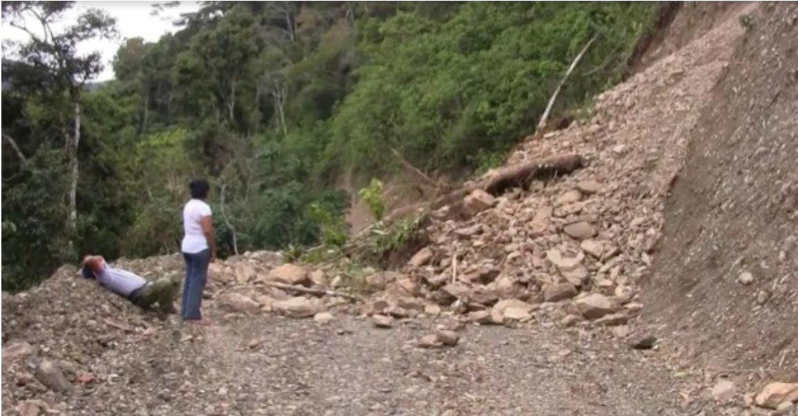
Figure 22: Edison, Gladys, and the author (not pictured) prepare to spend several hours clearing a small landslide on the road to Yokiri
