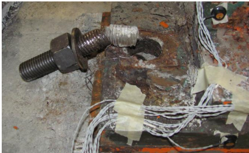
Figure 6.89 Photograph showing the severely deformed and fractured anchor bolt
