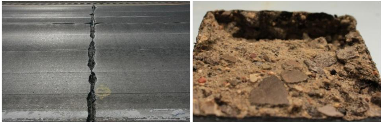
(a) Joint deterioration
