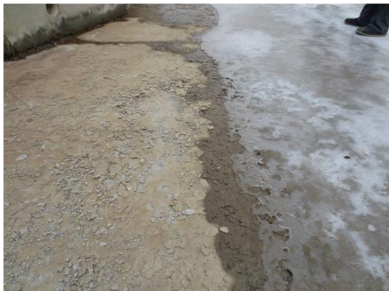
(c) Concrete slab surface scaling
