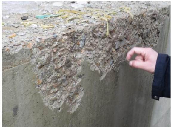
(b) Concrete spalling
