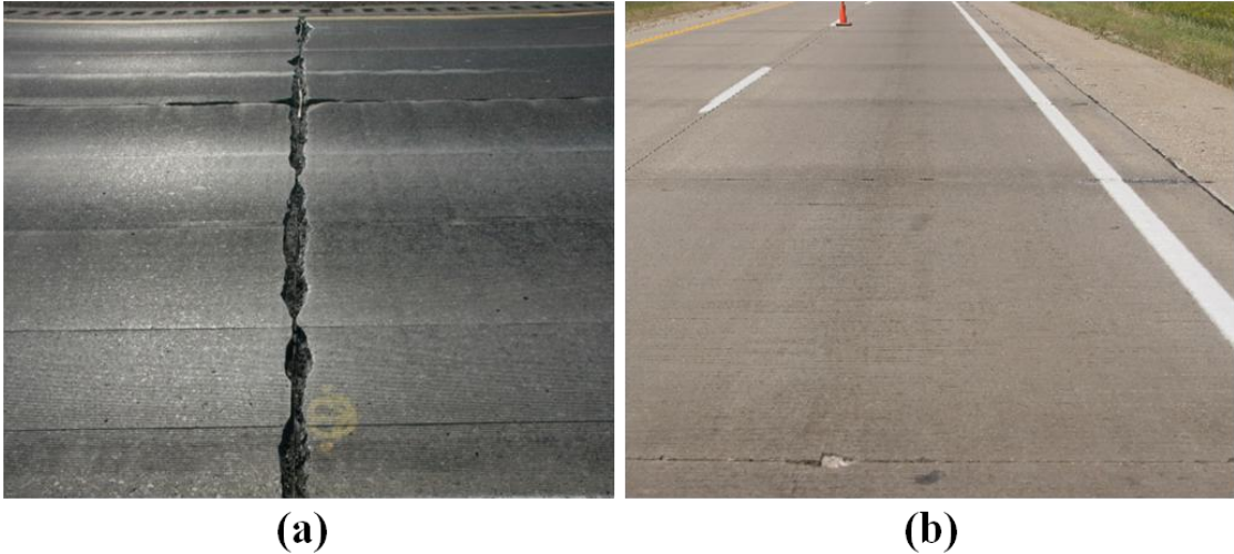
Figure 1.2 (a) Joint distress associated with salt frost deterioration and (b) transverse joint staining (by courtesy of Prof. Will Hansen)
