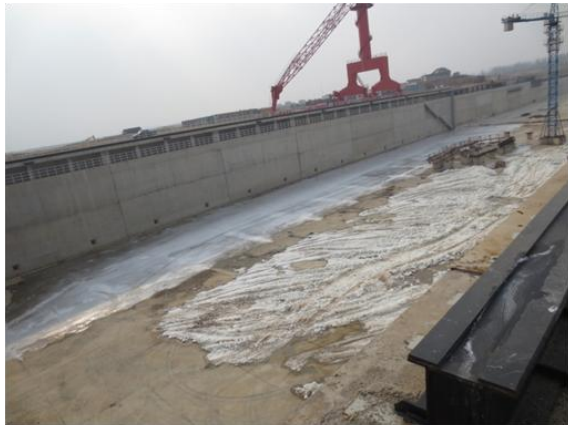
(a) Shipyard exposed to freezing and sea water
