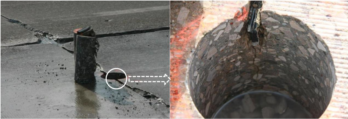
Figure 1.3 Joint spalling at the bottom of a saw-cut joint associated with deicer salt scaling (by courtesy of Prof. Will Hansen)
