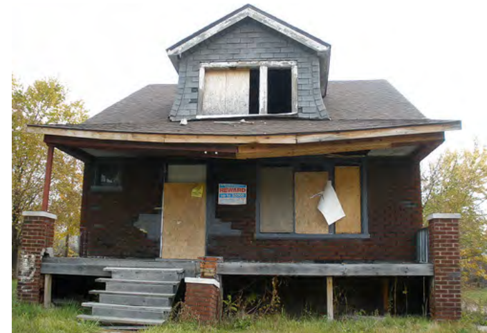
Figure 4.2: Home in great disrepair
