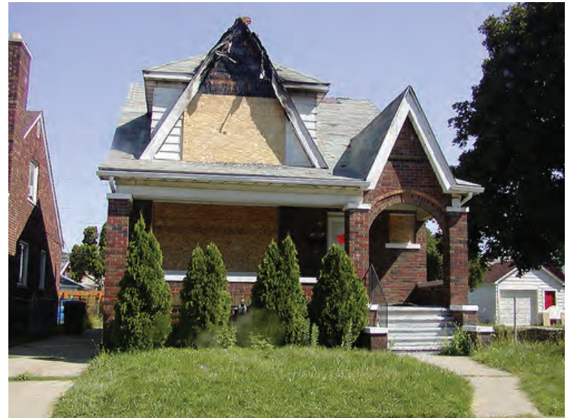
Figure 6.9 Candidate for demolition
