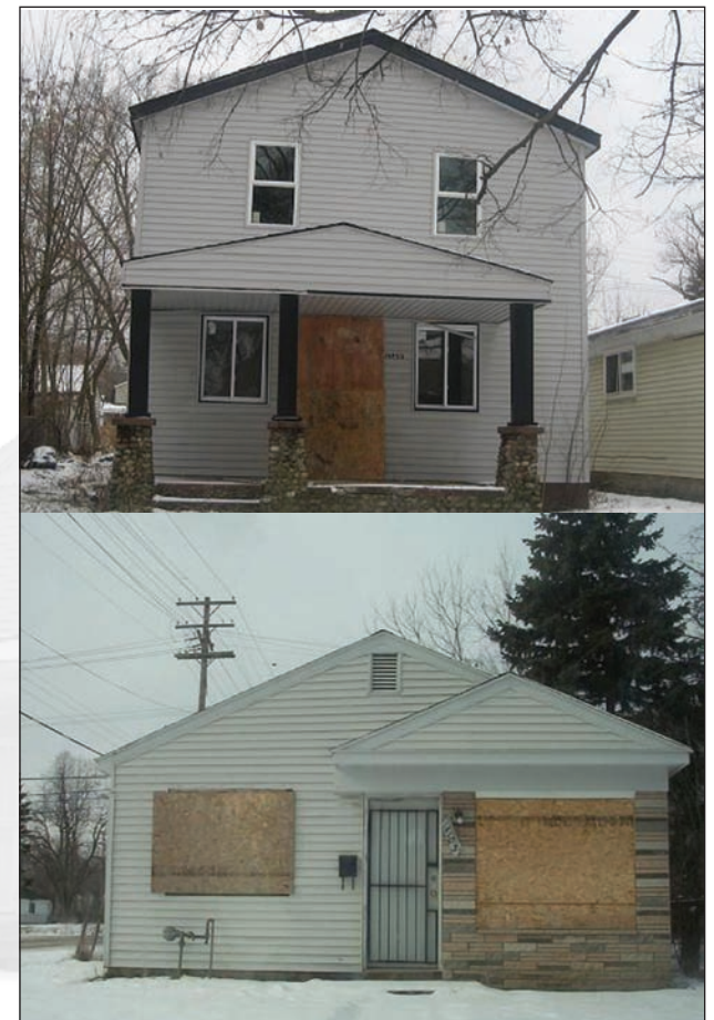
Figure 5.16: Examples of Boarded Unoccupied Houses with Good and Fair Physical Structure
