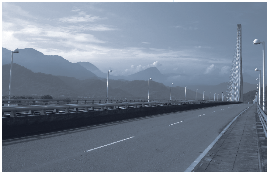
The Gi-Lu Bridge in Taiwan was instrumented in 2007 to collect and analyze ambient vibration data.
