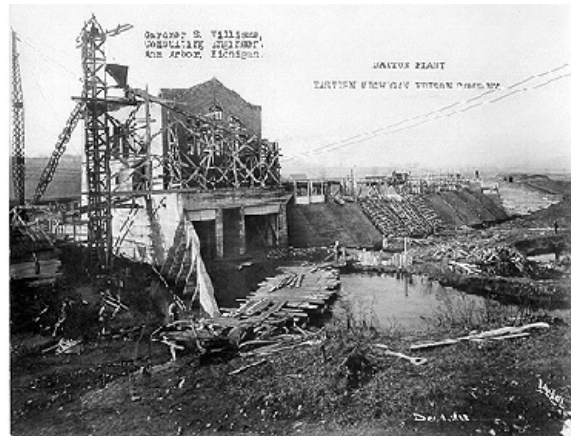
Barton Plant, Eastern Michigan Edison Co., Dec. 1, 1912 from Gardner Stewart Williams Papers
