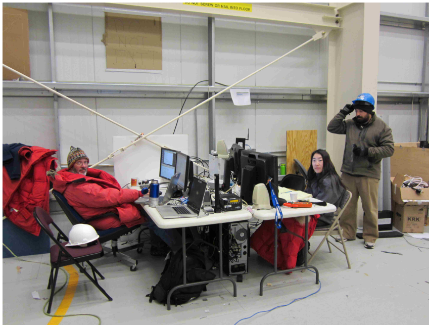
Figure 5.114: Jim Musser, Nahee Park and Myself after replacing one of CREST's two battery banks, which had been overcharged by a faulty charge controller.
