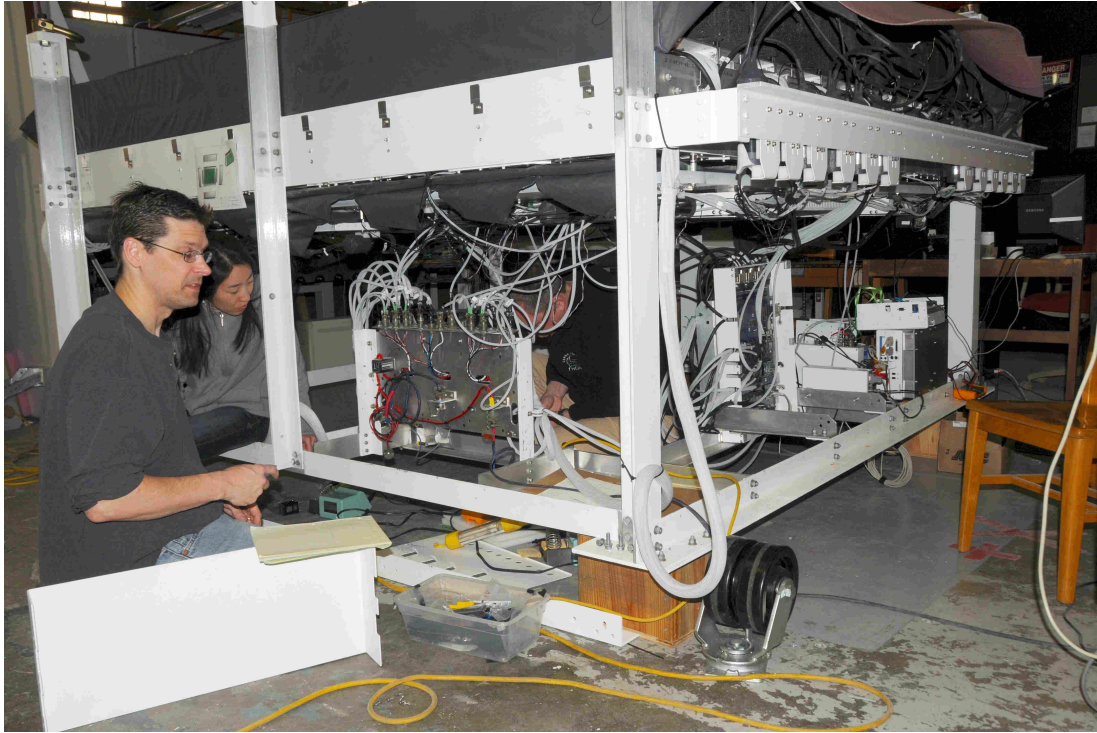
Figure 5.16: Scott Wakely, Nahee Park and Michael Schubnell install the power panel inside the CREST instrument. Photo courtesy of R. Northrop.
