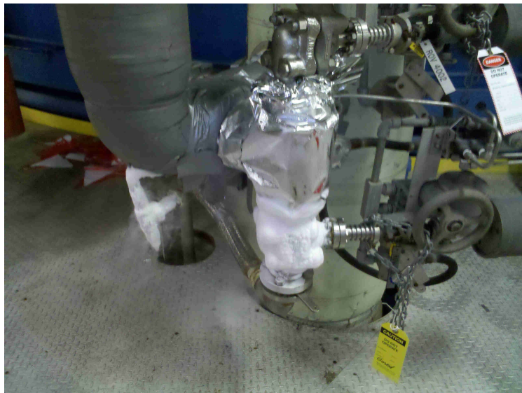
Figure 5.11: The LN 2 pipe which ruptured during the first cold fill. Due to Plum Brook's strict safety protocol (and the grace of God) no one was injured.
