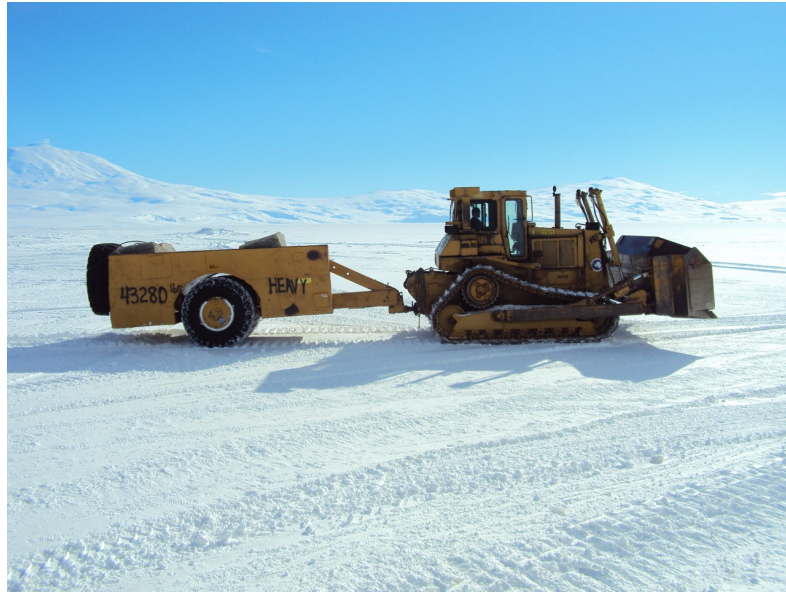
Figure 5.75: It turns out the best way to smooth an ice road is to roll a very, very heavy wagon on top of it.
