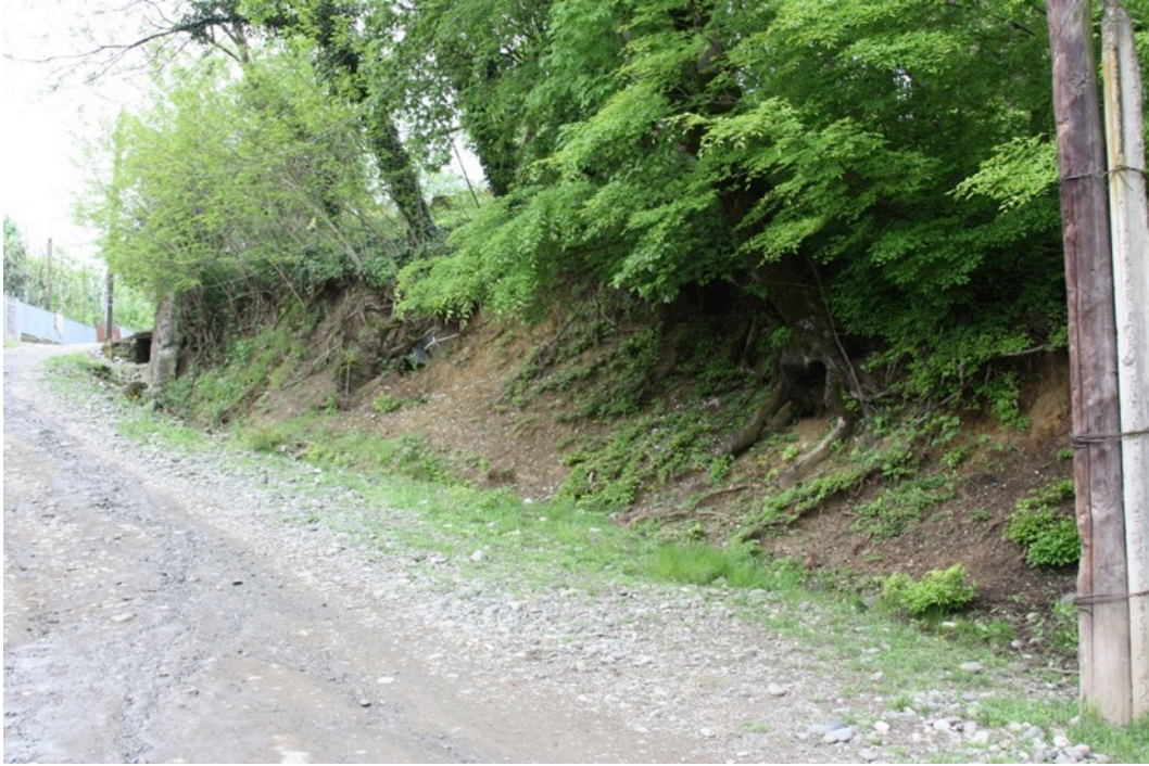
Figure A.10: Northern scarp of the road cut at E002. Photo by R. Hughes.
