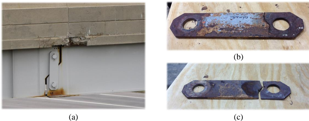
Figure 1-1. Pin and hanger detail: (a) suspending center span girder from end span girder and (b-c) extensive corrosion damage and section loss.
