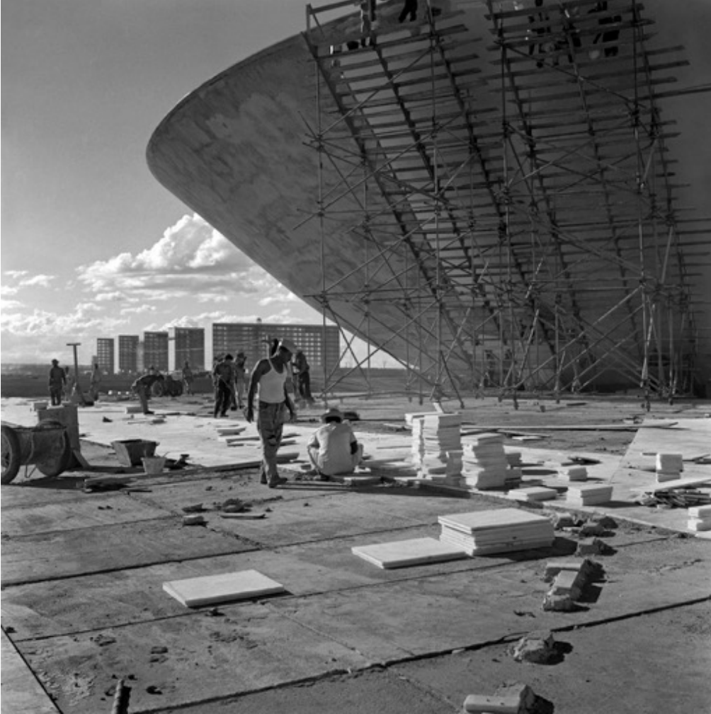
Image 7. Construction of Brasília, National Congress. Source: Marcel Gautherot, ca. 1959, Instituto Moreira Salles.
