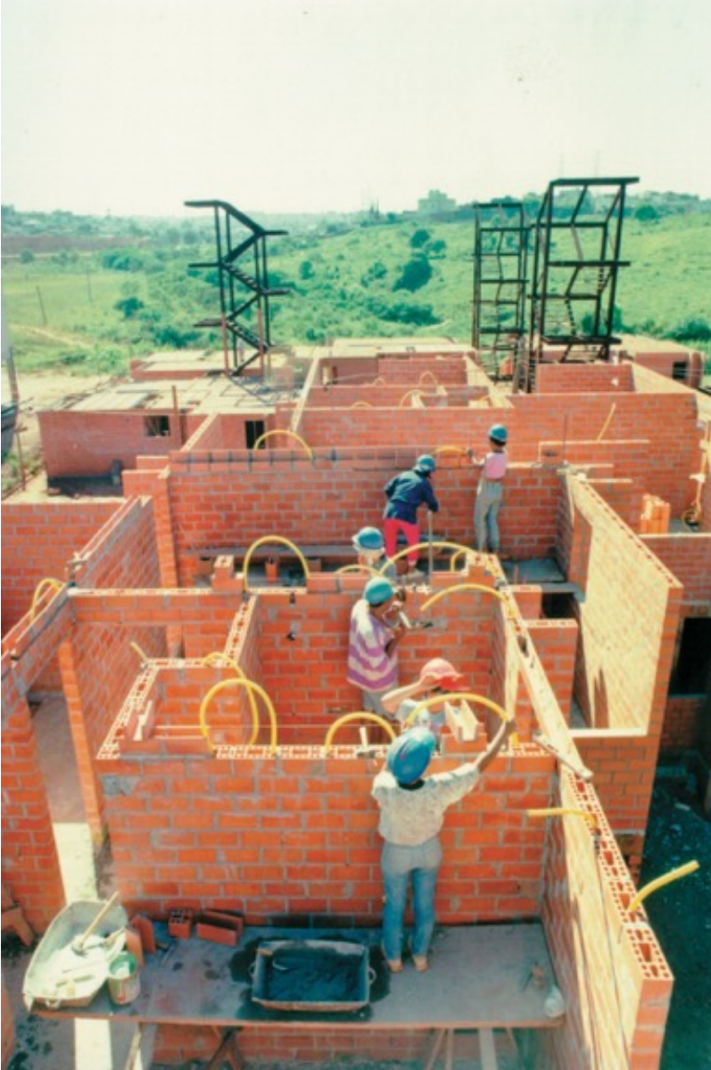
Image 33. Construction of the Talara housing complex by a self-build cooperative. Usina coordinated the participatory design and construction of this housing complex. In this image, it is possible to see the combination of the work of future residents using a more traditional construction material (structural brick) and prefabricated components (metallic stairs). Source: Usina.
