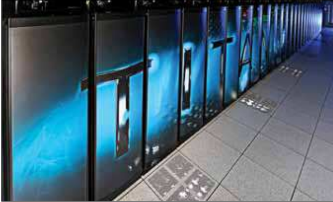
Titan supercomputer (Oak Ridge National Laboratory)
