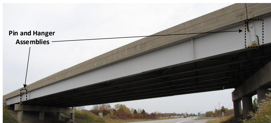
Figure 2.7, Side view of the Telegraph Road Bridge located in Monroe, MI (pin and hanger connections are pointed out in the figure)
