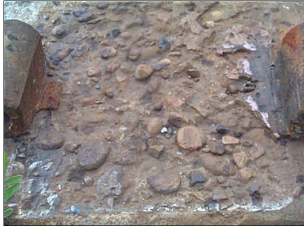
Figure 8.2: Erosion of cement paste on the rail seat of a prestressed concrete tie. 13
