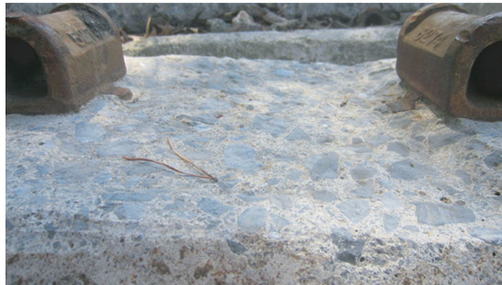
Figure 8.3: Severe RSD including erosion of cement paste and aggregate. 14
