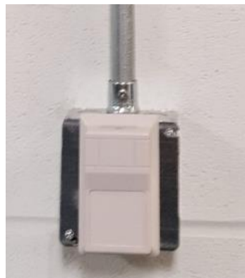
Figure 22: Thermostat that measures hot and cold aisle temperature
