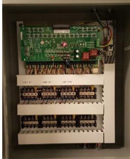
Figure 19: Process controllers connecting power meters
