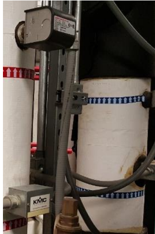
Figure 21: Temperature sensors for hot and cold coils
