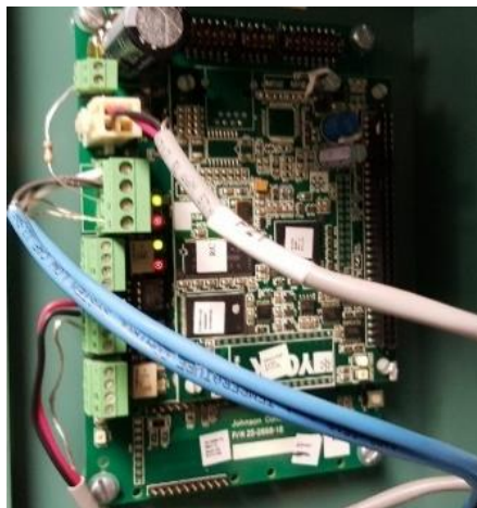
Figure 20: On board chiller control board
