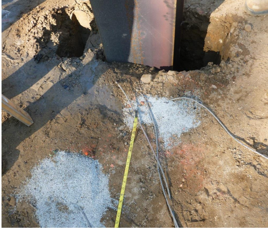
Figure 5-17 Conductor cables coming out on the ground surface
