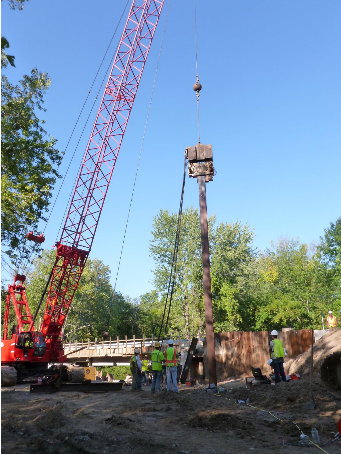
Figure 6-13 Extraction of test pile with vibratory hammer after the end of monitoring the installation process with the diesel hammer
