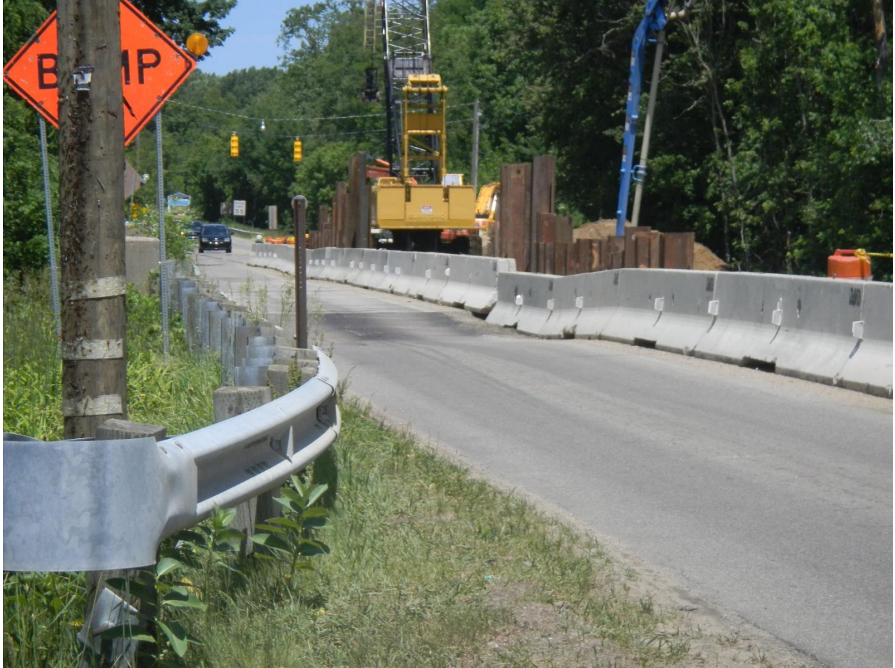
Figure 6-40 Bump created on the road close to pile driving operations at M-139 site
