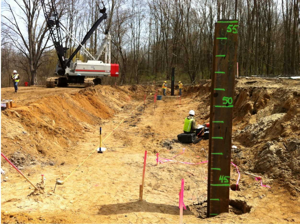
Figure 6-15 Tested piles #1 (front) and #18 (back) after the end of driving at US-131 site at bridge abutment A
