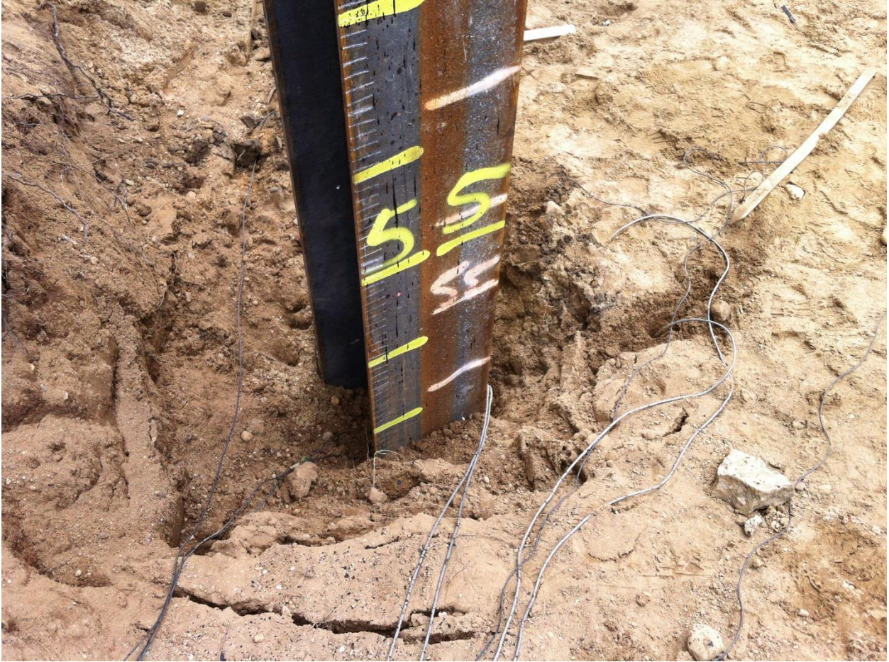
Figure 6-161 Settlement around pile 54 after the end of driving at US-131 B site
