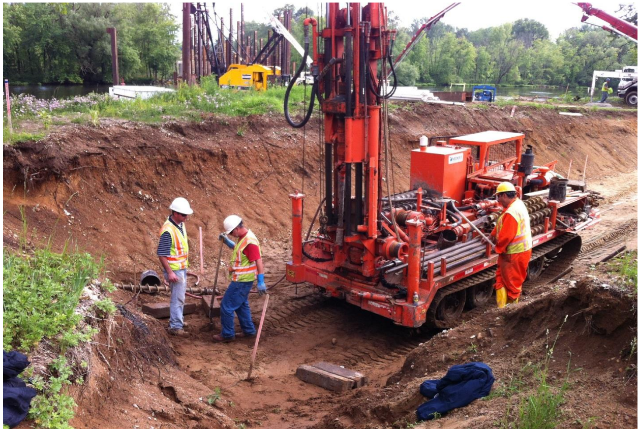
Figure 5-11 View of drill rig used to push sensor cones in desired depths
