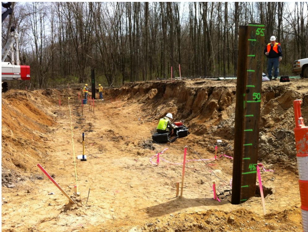
Figure 6-122 Abutment A after the end of driving pile 1 (front) and pile 18 (back)
