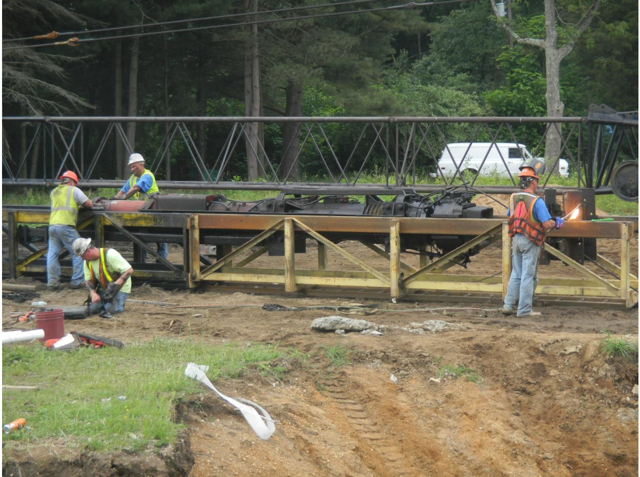
Figure 6-16 Lead and hammer preparation before pile driving at US-131 site at bridge abutment B
