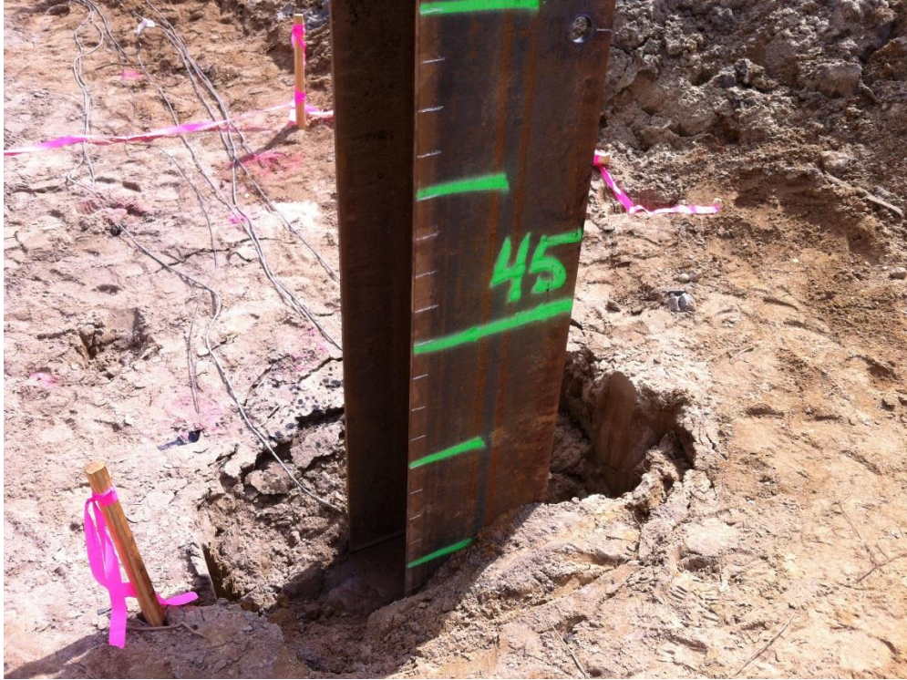
Figure 6-123 Settlement around pile 1 after the end of driving at US-131 A site
