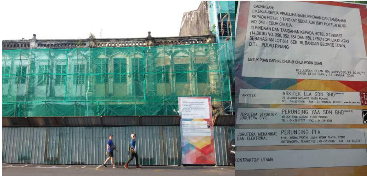
Figure 5.5: View of the five shophouses in Chulia Street in May 2015 (author's photograph)
