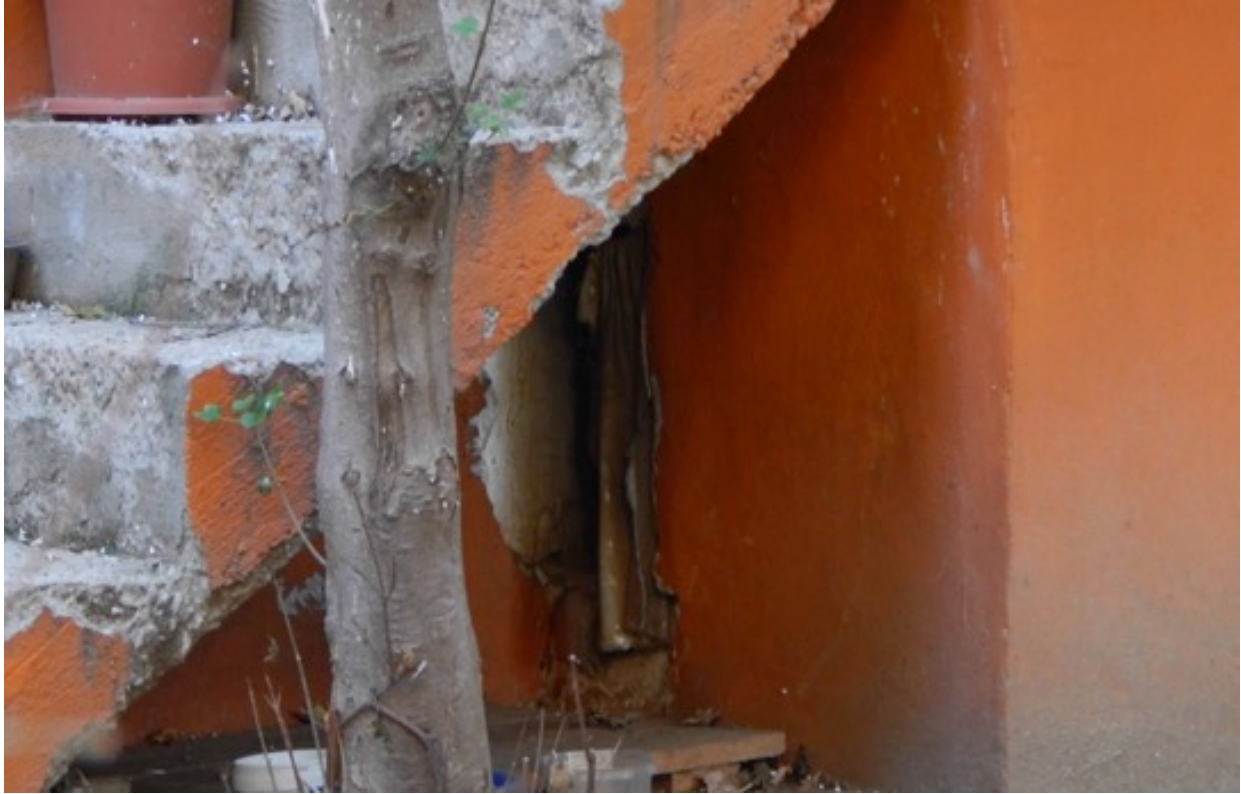
Figure 42: Close up of secret passage to the basement under the concrete staircase.
