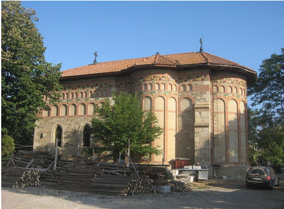
Figure 3.57 Church of the Beheading of St. John the Baptist, Vaslui, Moldavia, 1490, view from S (source: Cezar Suceveanu)
