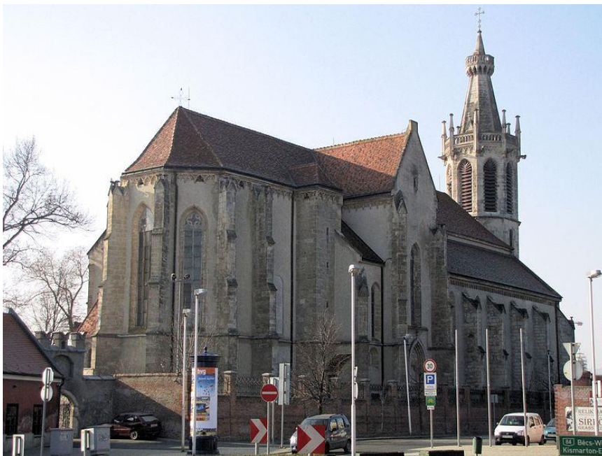
Figure 3.94 Exterior buttresses, Parish Church of St. Michael, Sopron, Hungary, last quarter of the thirteenth century, view from NE (source: Kovacs Daniel)
