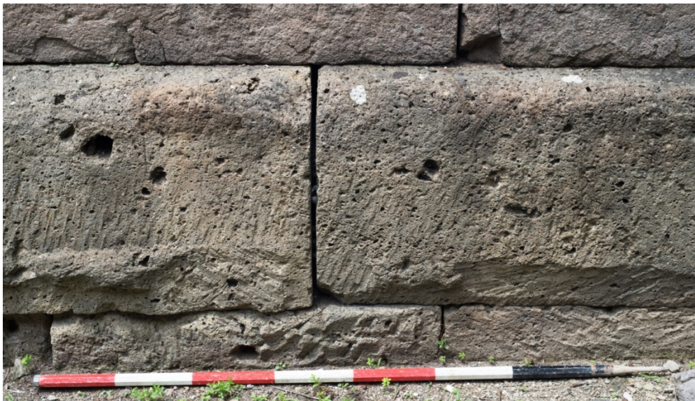
Figure 24: Tufo Giallo blocks in foundation of eastern edge of Republican podium, showing tool marks and remainder of roughly dressed surface (left block) indicating contemporary ground level. 1.6 m scale (author).
