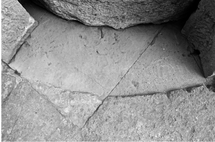
Figure 60: Smoothly-dressed surface cut into Anio block pavement for insertion of circular monument (author).
