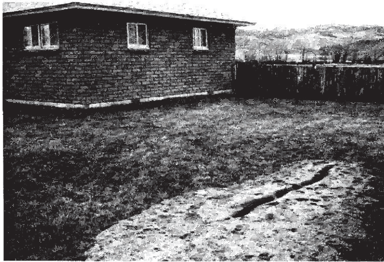
Figure 2.36: Ejected soils, including sand and gravel, observed following the 1983 Borah Peak earthquake ( Youd et al. , 1985)
