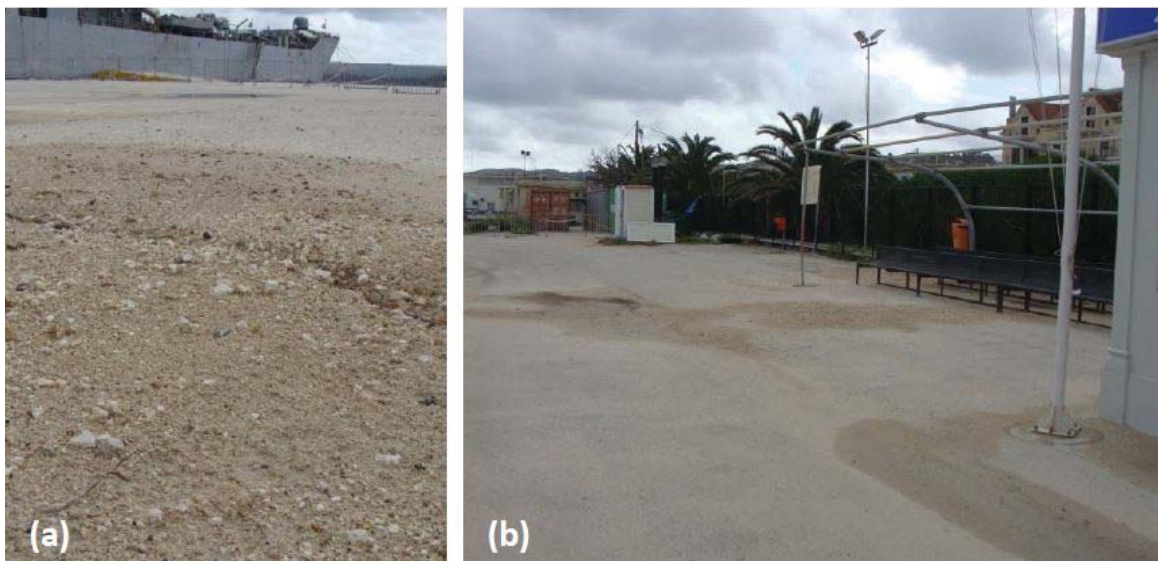
Figure 6.73: Liquefaction observed in Argostoli following 2014 Cephalonia earthquakes (Nikolaou et al. , 2014)
