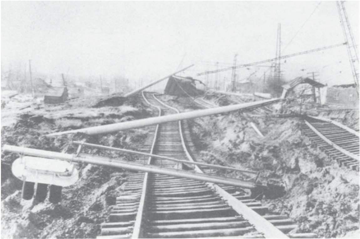
Figure 2.46: Liquefaction of railway embankment, 1988 Armenia earthquake (Yegian et al. , 1994)
