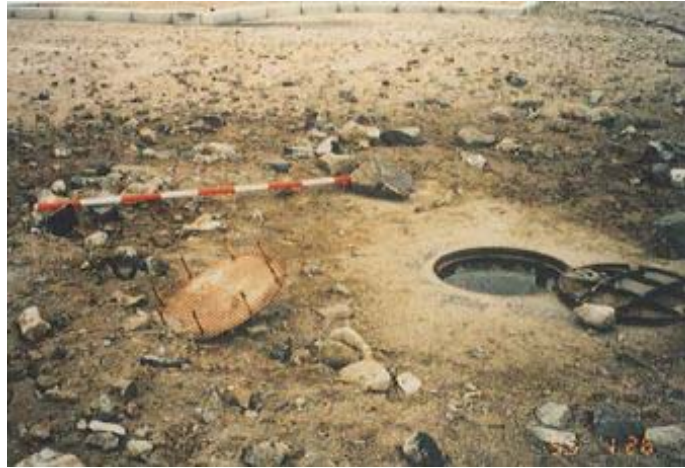
Figure 2.49: Observed gravelly soils ejected from the ground during liquefaction, 1995 Kobe earthquake ( Hamada, 2014 )
