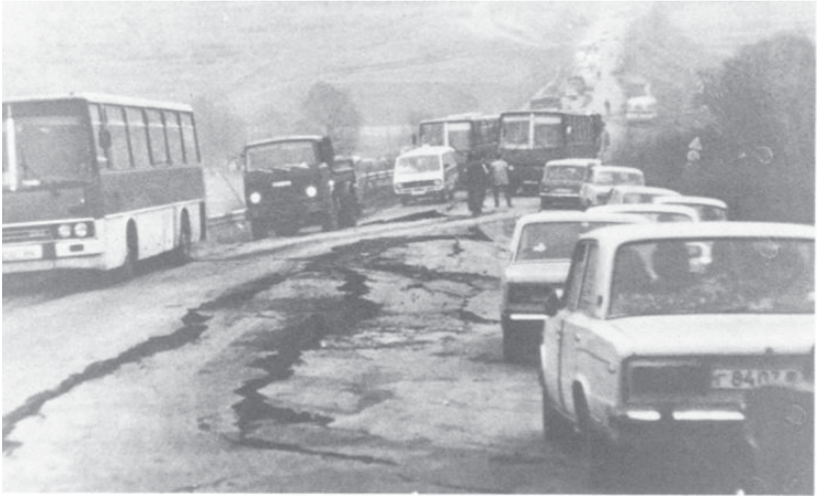
Figure 2.42: Liquefaction of roadway embankment, 1988 Armenia earthquake ( Yegian et al., 1994 )
