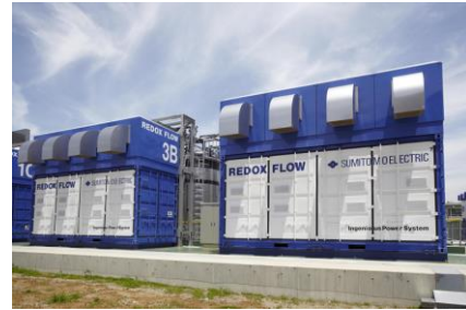
Figure 1-1. Sumitomo Electric Industries redox flow battery [5]
