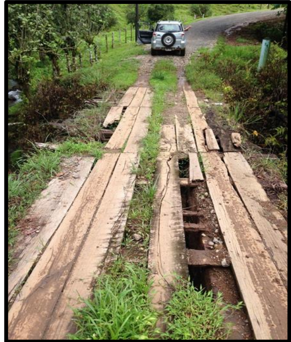
Figure 3.3: Bridge conditions were highly variable and at times necessitated longer alternative routes.
